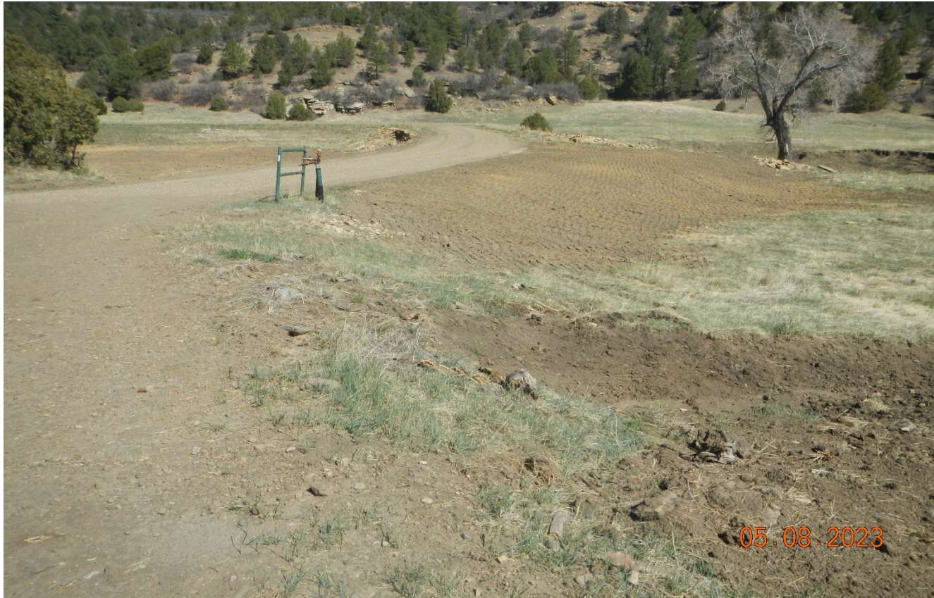
Photo 2. Facing back northwest toward the stream crossing repair. Disturbed areas were seeded and hydromulched.
