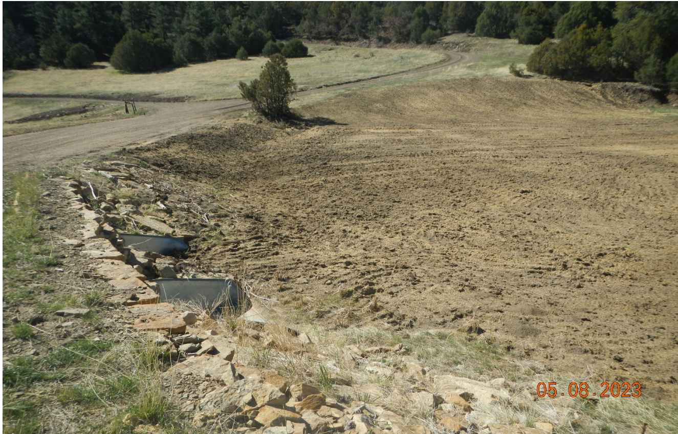
Photo 1. Facing south along the road at the stream crossing. The culverts have been repaired and bank was regraded. Disturbed areas were seeded and hydromulched.
