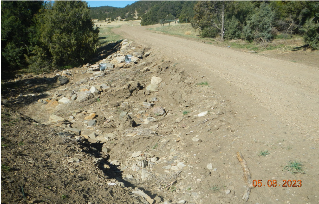
Photo 1. There is erosion along the access road at this drainage crossing Lat/Long:37.05023,-104.66580. This embankment needs to be stabilized.
