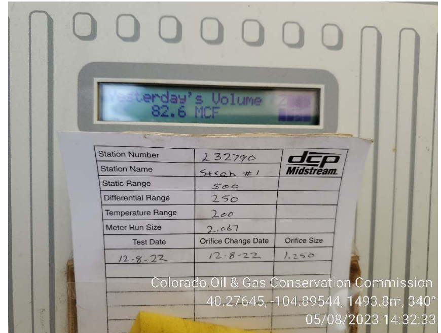
DCP gas sales meter calibration card and previous day product sold volume.
