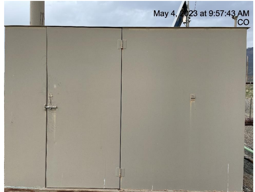
Photo # 6929 Meter calibration info not conspicuously posted
