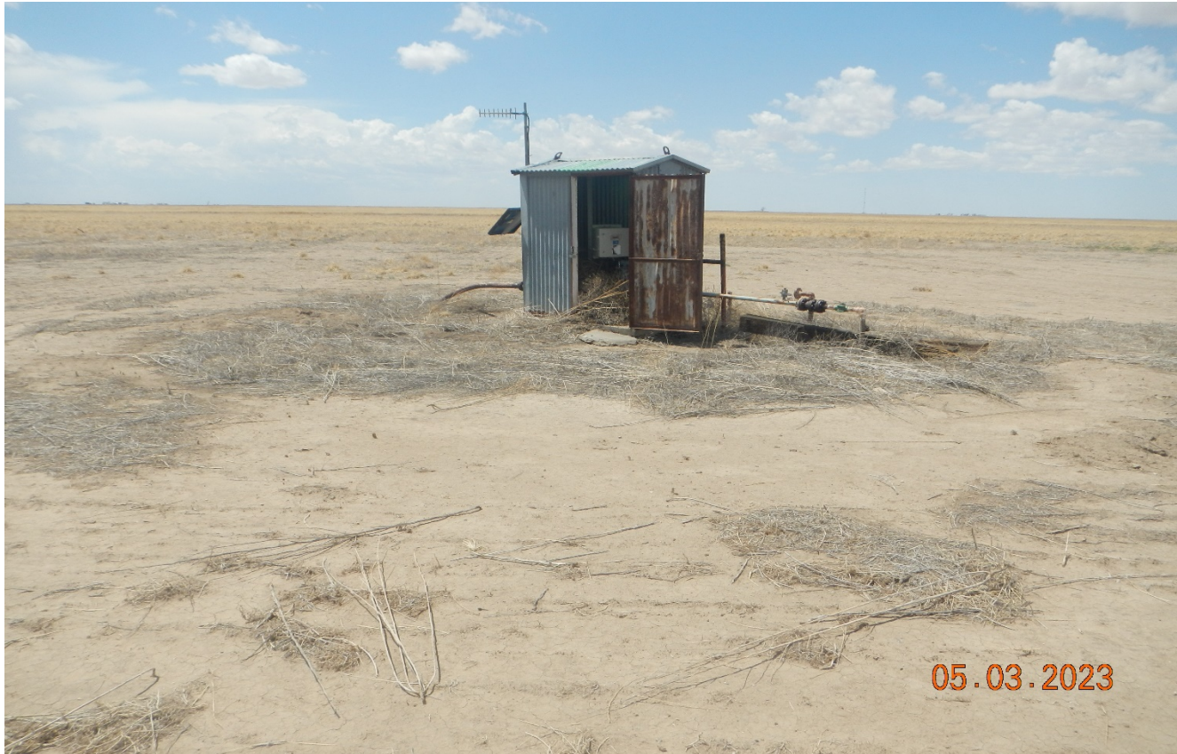
Photo 1. The meter run still remains at the location. All equipment should have been removed within 3 months of abandonment.
