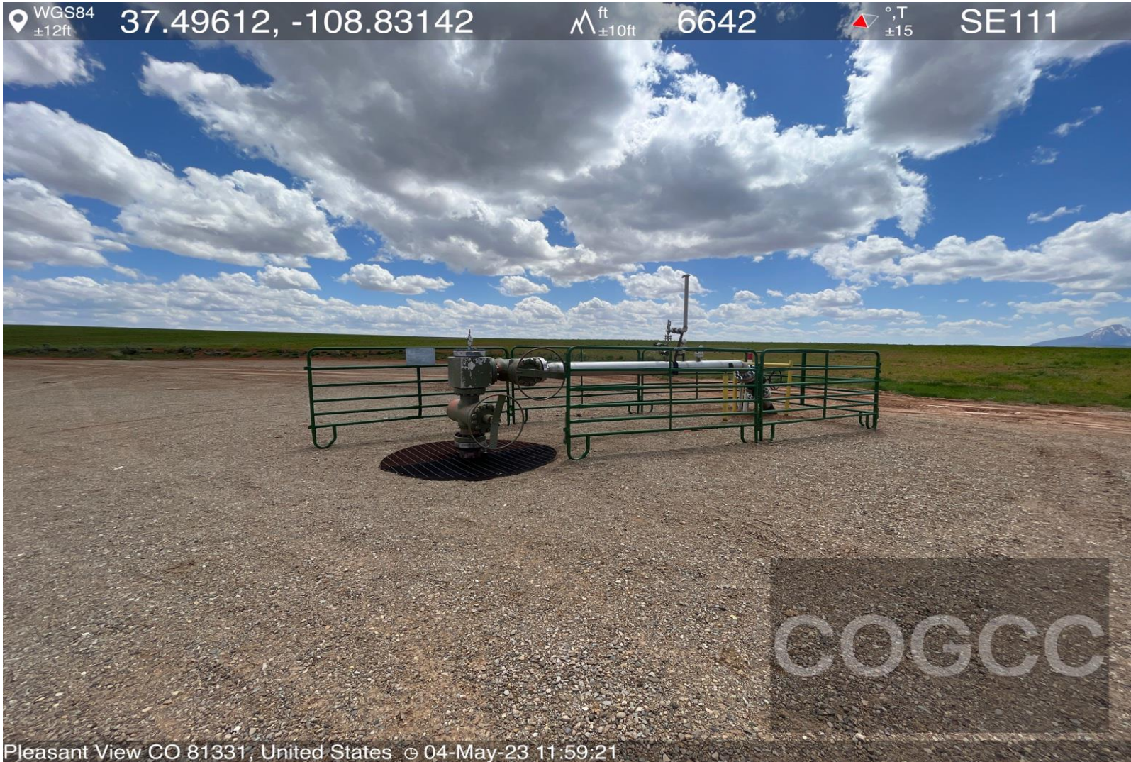
Photo #2 View of wellhead and flowline assembly.
