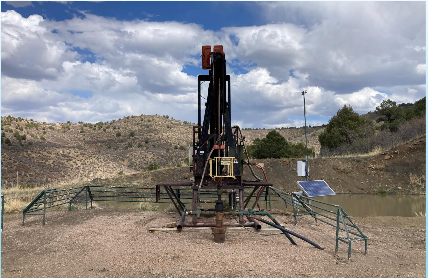
PHOTO 2: WELLHEAD AND EQUIPMENT
