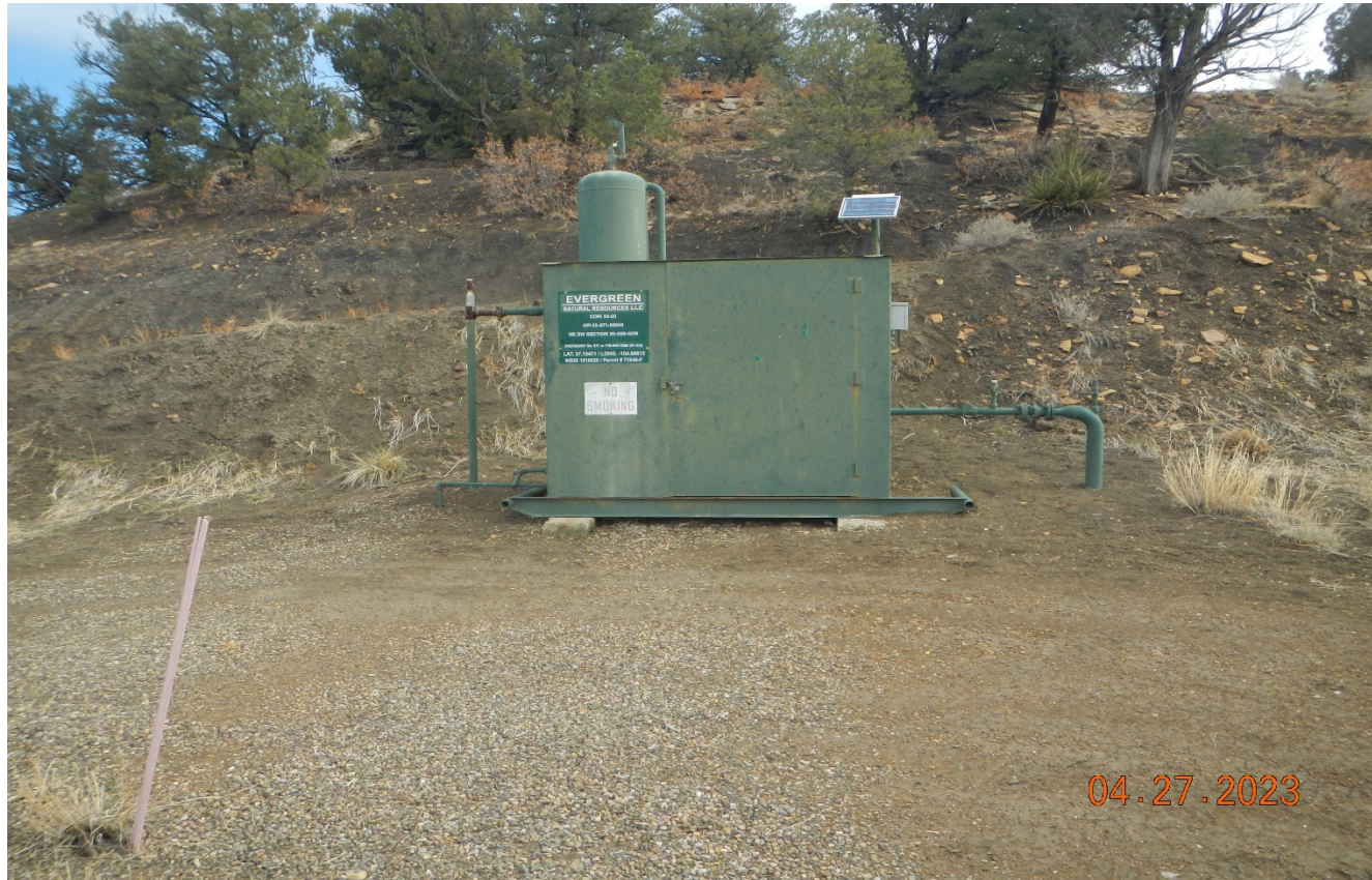
Photo 3. Sign is posted at meter shed.
