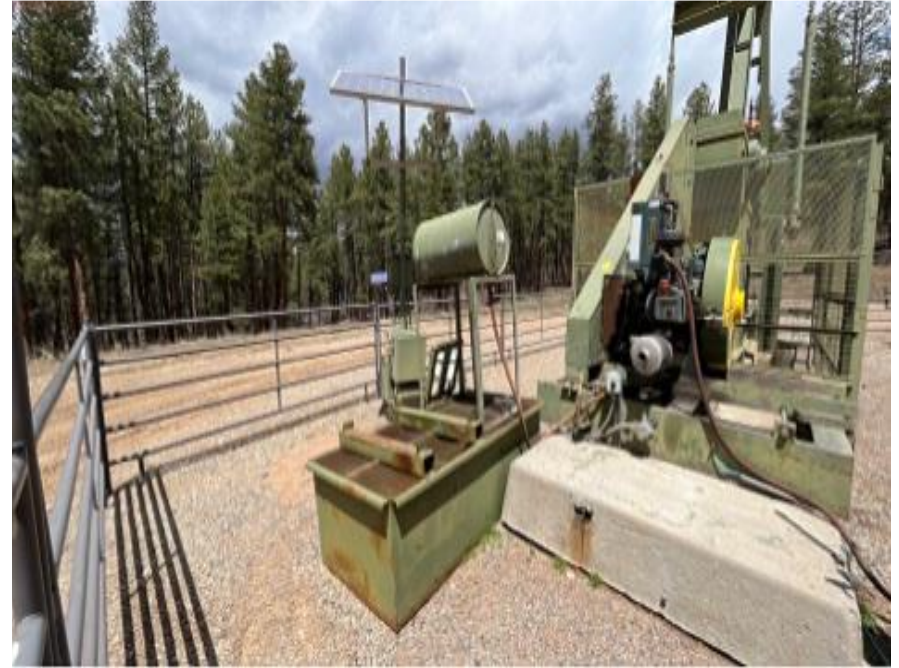
Photo #2. View of wellhead tank and spill containment.
