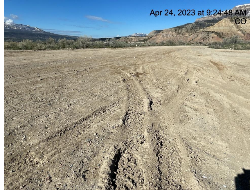
Photo # 6107 Lack of stabilization/Compaction on location
