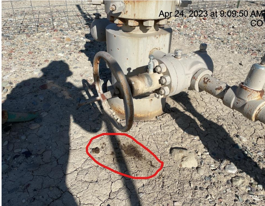
Photo # 6074 Stained soils
