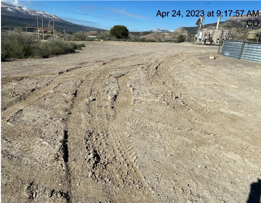
Photo # 6089 Lack of stabilization/Compaction/Insufficient tracking BMP's
