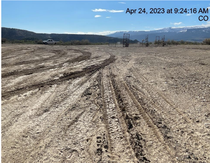
Photo # 6105 Lack of stabilization/Compaction on location
