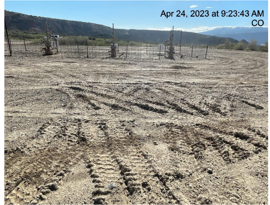
Photo # 6104 Lack of stabilization/Compaction on location
