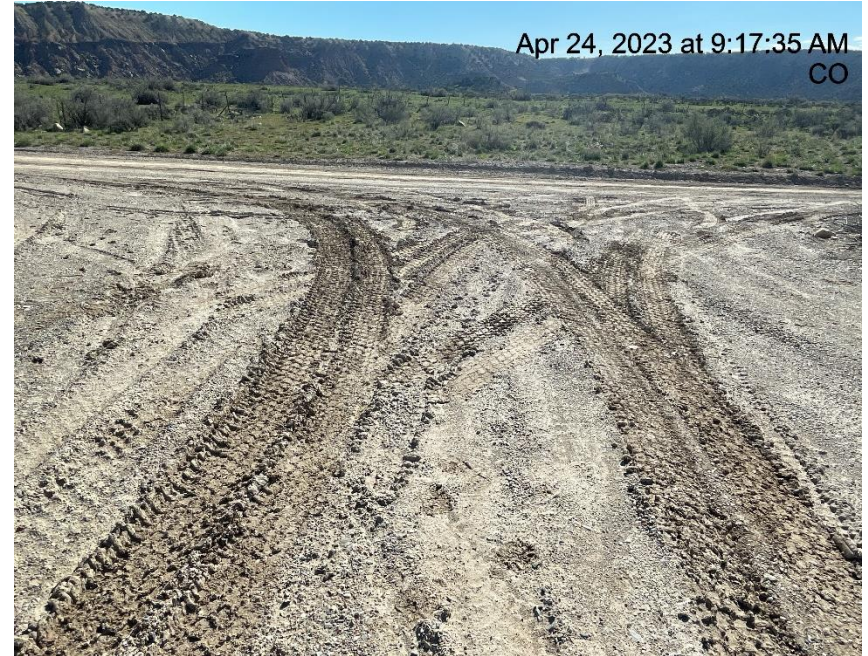
Photo # 6088 Lack of stabilization/Compaction/Insufficient tracking BMP's
