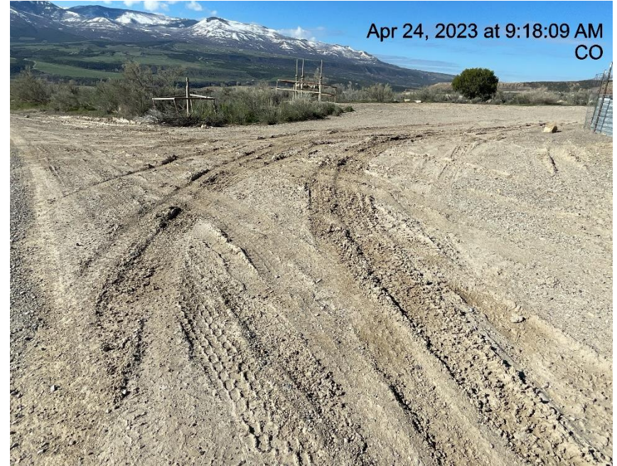
Photo # 6090 Lack of stabilization/Compaction/Insufficient tracking BMP's
