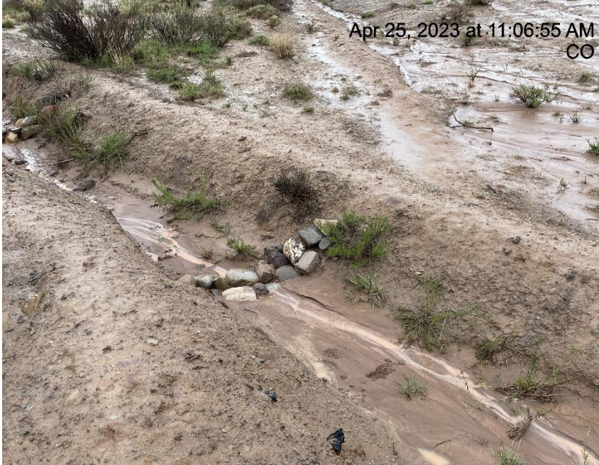
Photo # 6372 Check dams need maintenance
