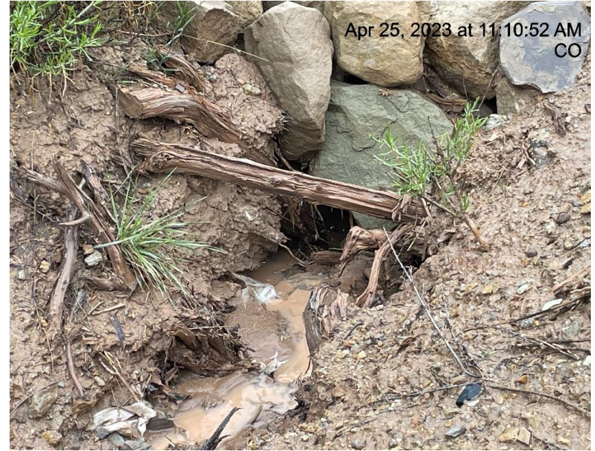
Photo # 6379 Rip Rap needs maintenance (near culvert at entrance to location)
