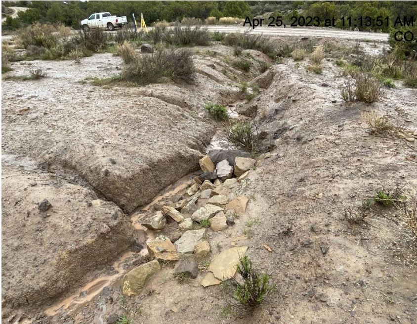
Photo # 6387 Erosion on slope going into ditch
