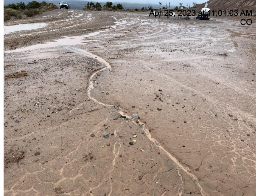
Photo # 6357 Erosion & transport of sediment on location (E/NE area of location)
