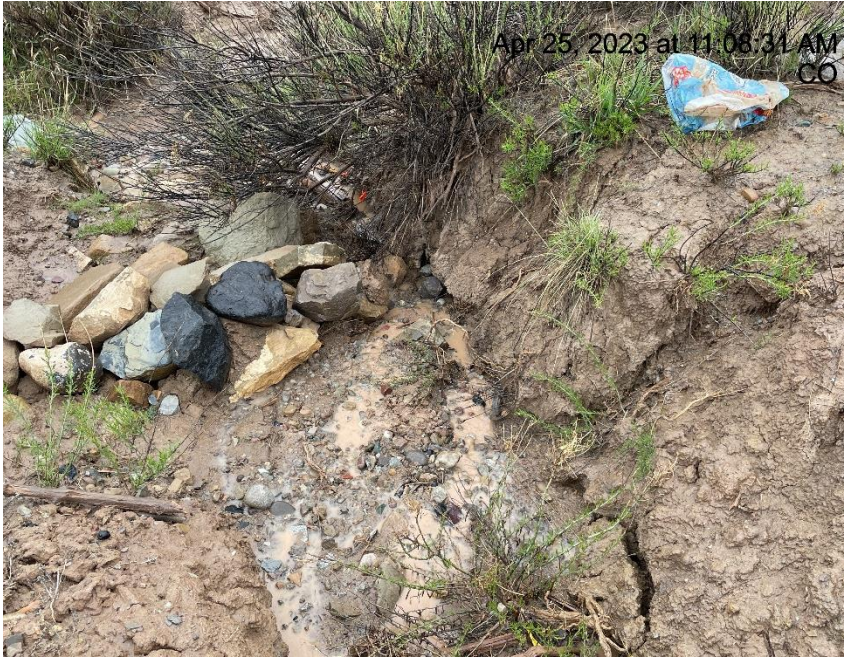
Photo # 6374 Ditch & Rip Rap need maintenance (near culvert at entrance to location)
