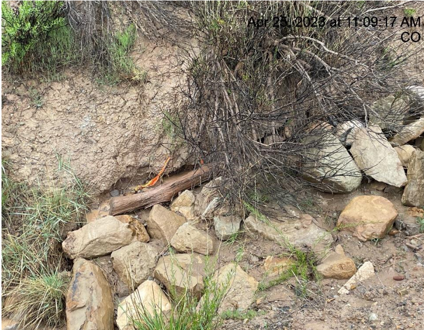
Photo # 6376 Rip Rap needs maintenance (near culvert at entrance to location)
