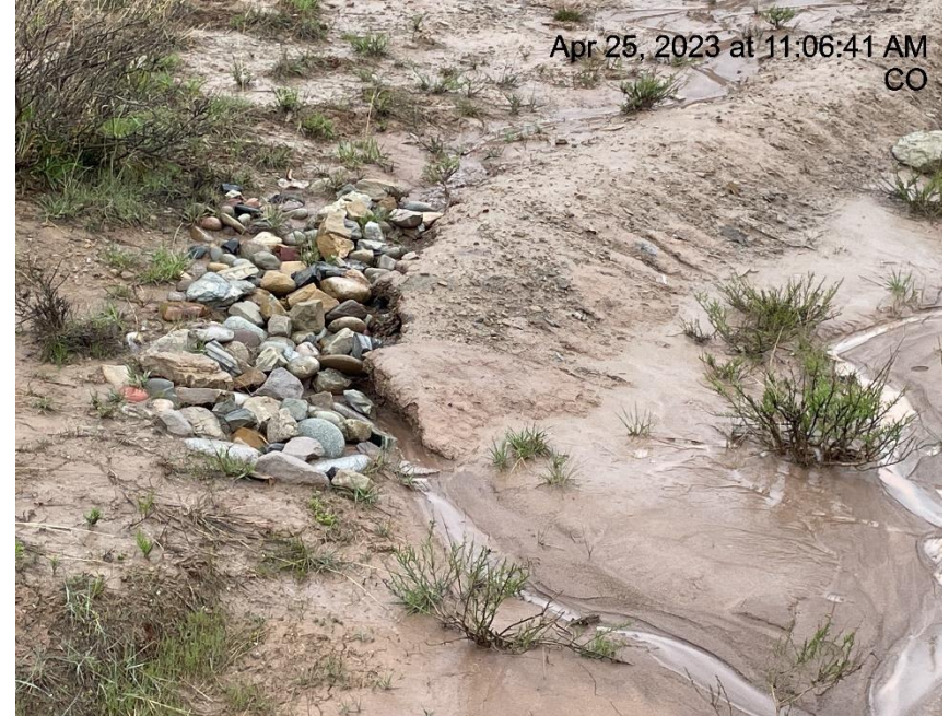
Photo # 6373 Rip Rap run needs maintenance
