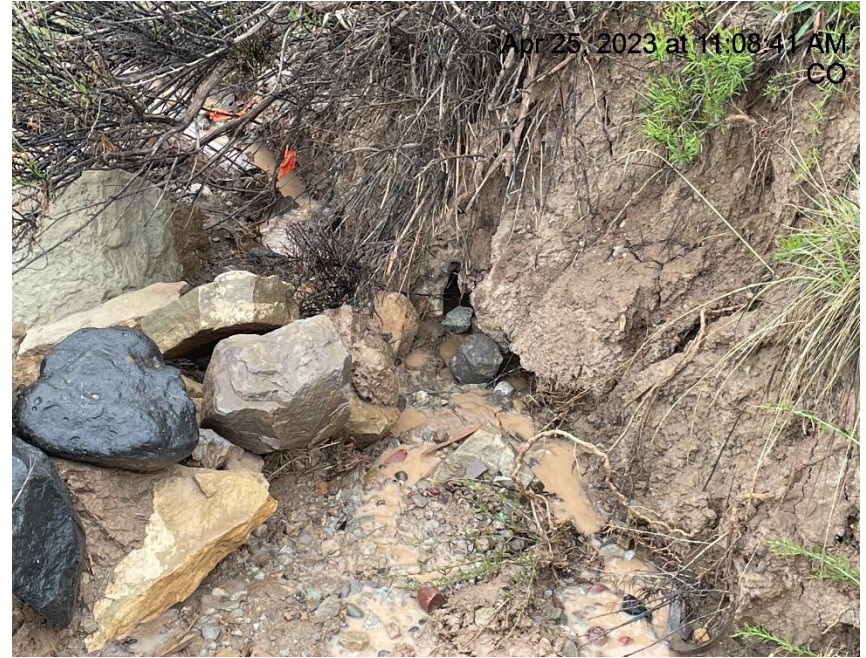
Photo # 6375 Ditch & Rip Rap need maintenance (near culvert at entrance to location)
