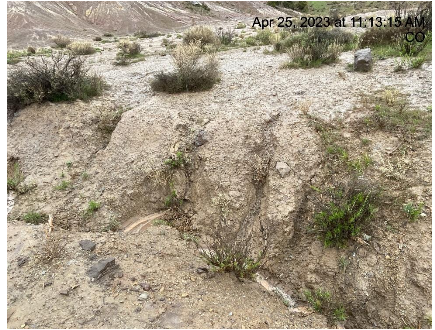
Photo # 6386 Erosion in multiple spots on slope of ditch
