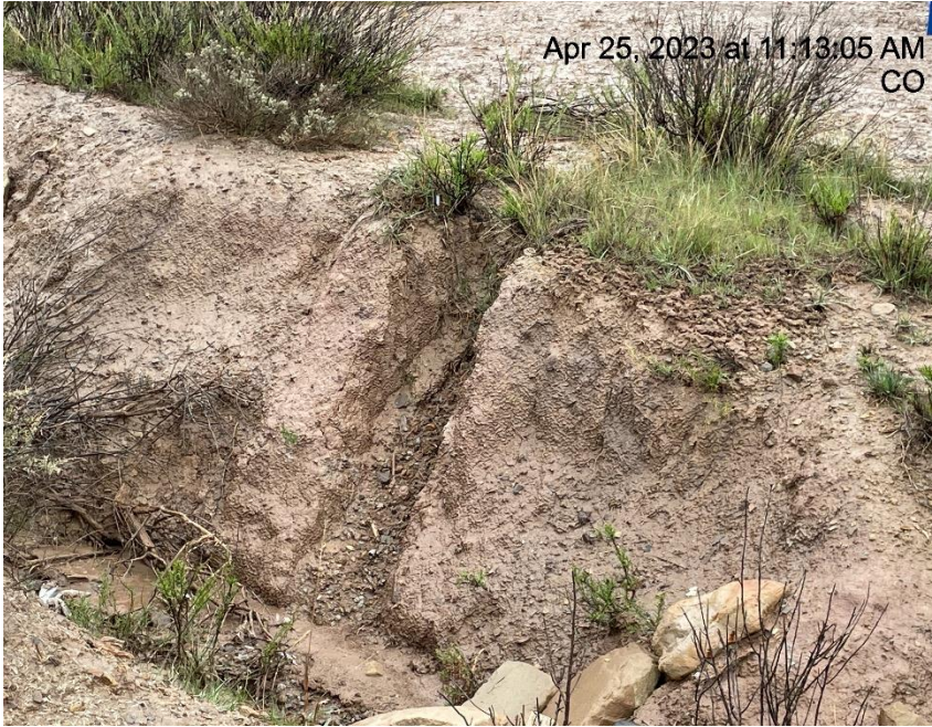
Photo # 6385 Erosion on slope of ditch near Rip Rap
