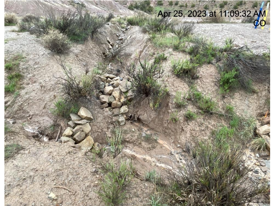
Photo # 6377 Rip Rap needs maintenance (near culvert at entrance to location)
