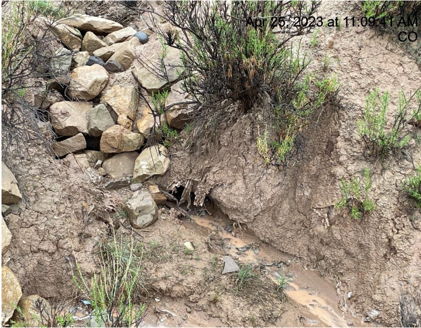
Photo # 6378 Rip Rap needs maintenance (near culvert at entrance to location)
