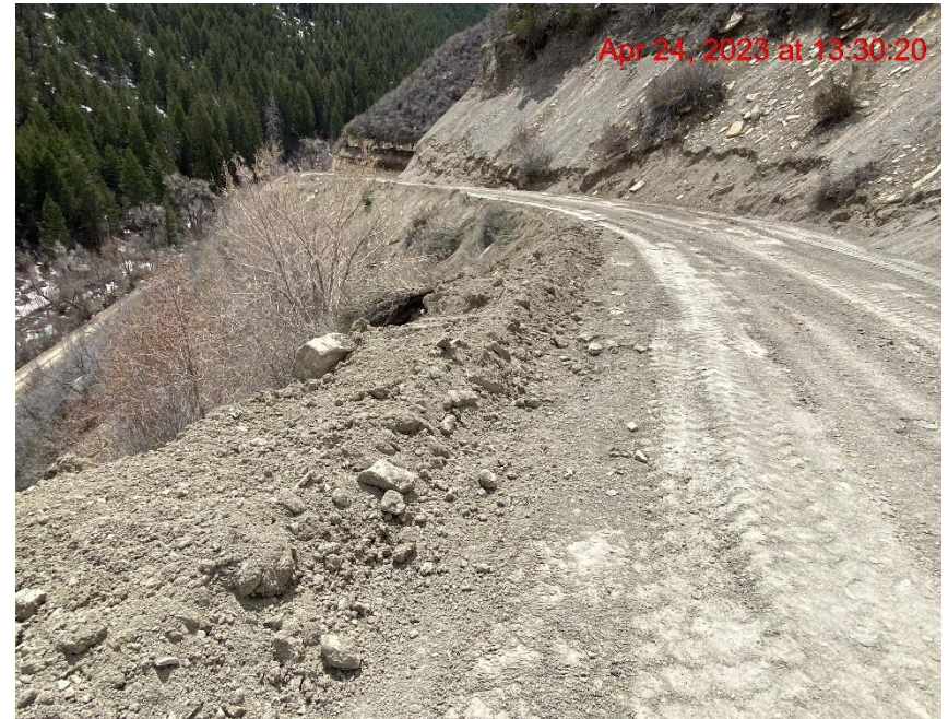
Access Road Degradation/Transportation of Sediment – Photo #02498
