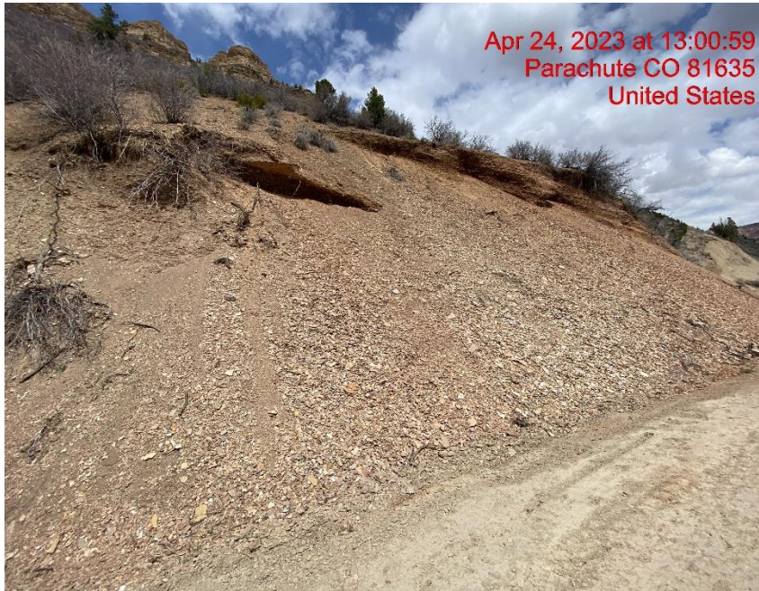
Cut Slope Erosion onto Access Road – Photo #02479
