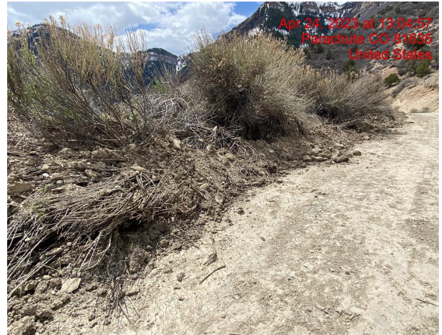
Access Road Degradation/Transportation of Sediment – Photo #02483
