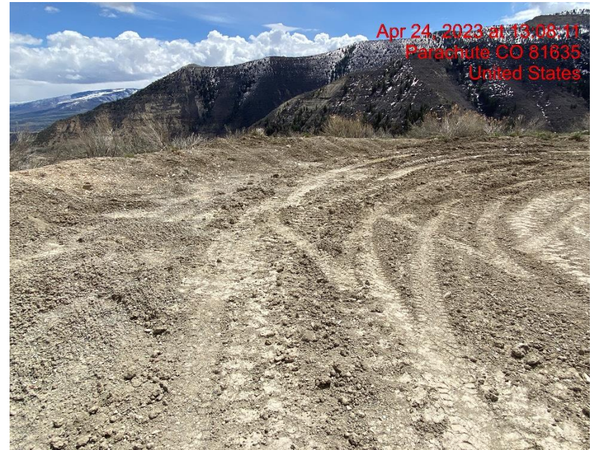
Lack of Stabilization – Photo #02488
