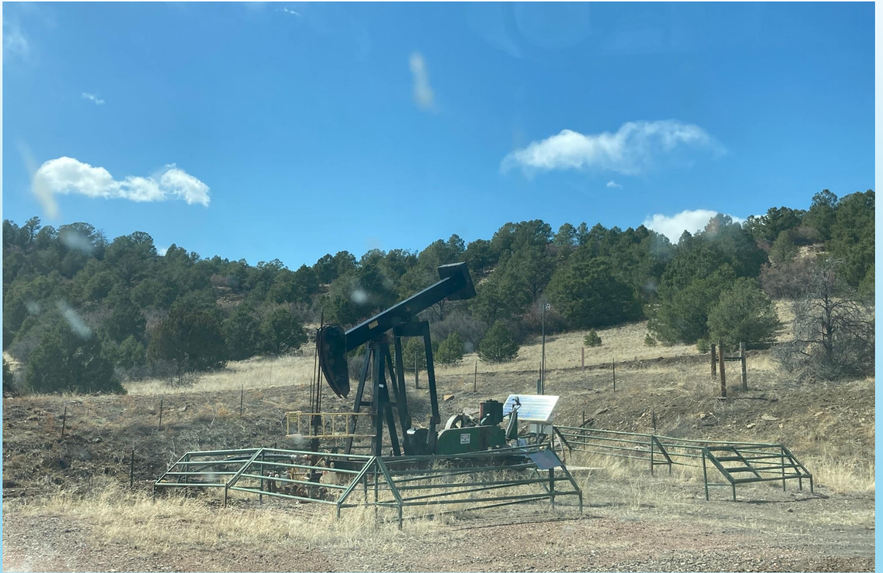
PHOTO 3: WELLHEAD AND EQUIPMENT
