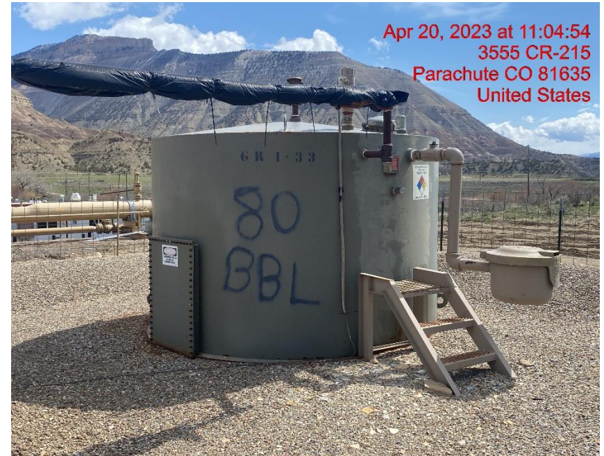
Tank Battery – Photo #02377
