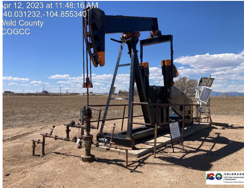
Pic 1 wellhead / Pump jack, no motor installed.
