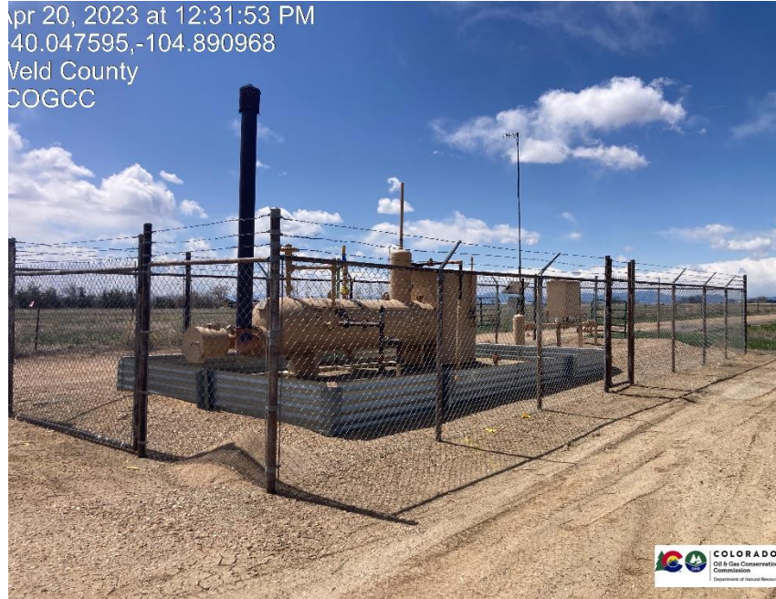
Pic 3 Separator, GMR, automation.
