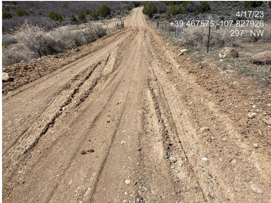
Photo 3. Photo shows the access road directly to the north of the location shows signs of lack of stabilization.
