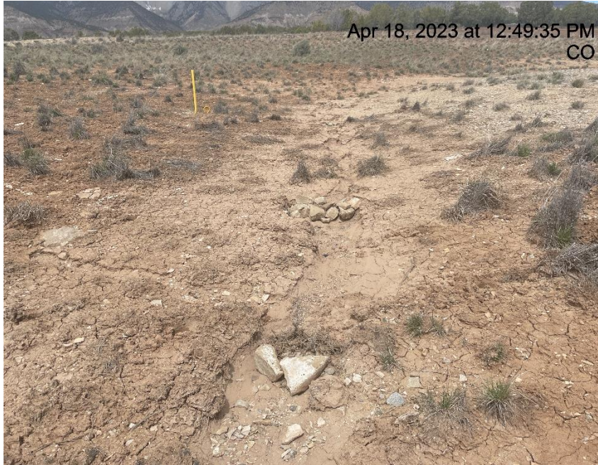
Photo # 5632 Check dams need maintenance (SW area of pad)
