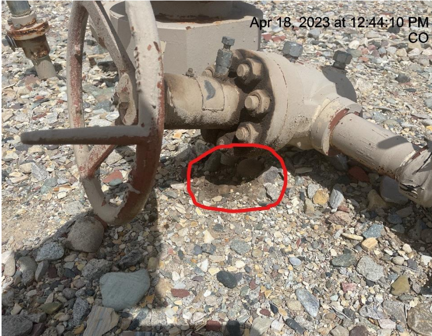
Photo # 5620 Stained soils & gravel
