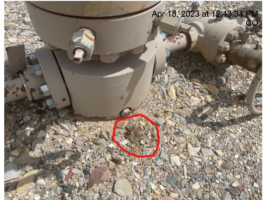
Photo # 5618 Stained soils & gravel
