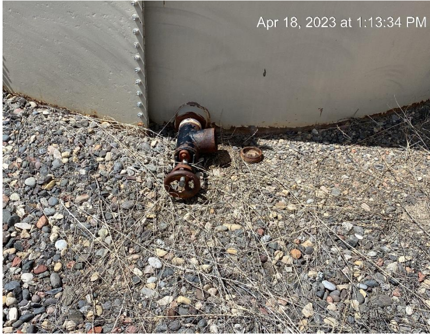
Open end tank valve
