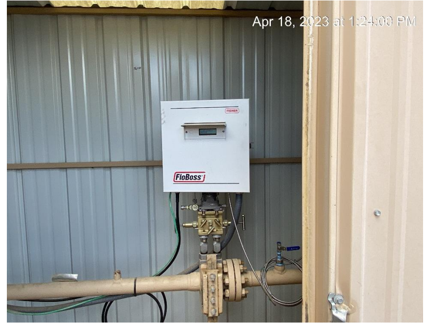
Gas meter calibration cards not visibly displayed
