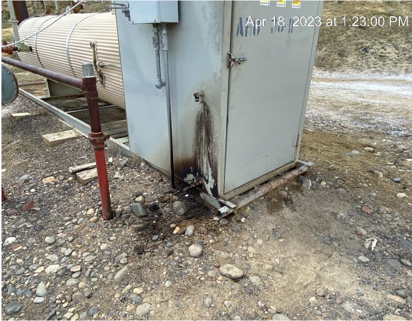
Equipment and soil staining
