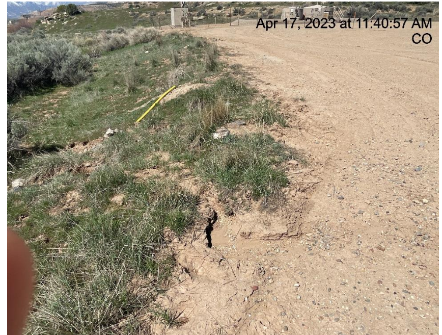
Photo # 5466 Erosion & transport of sediment off location (SE area of location, near entrance to location)
