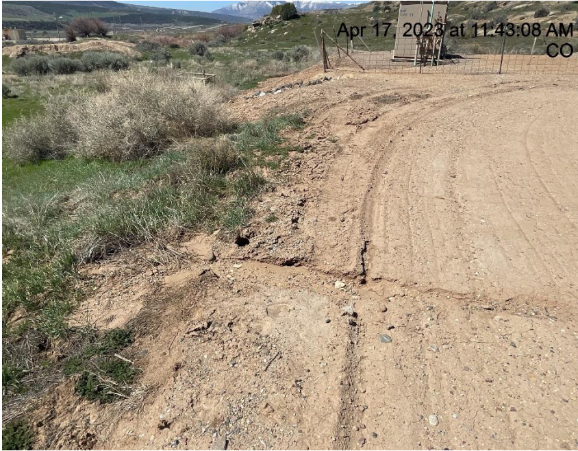
Photo # 5475 Erosion & transport of sediment off location
