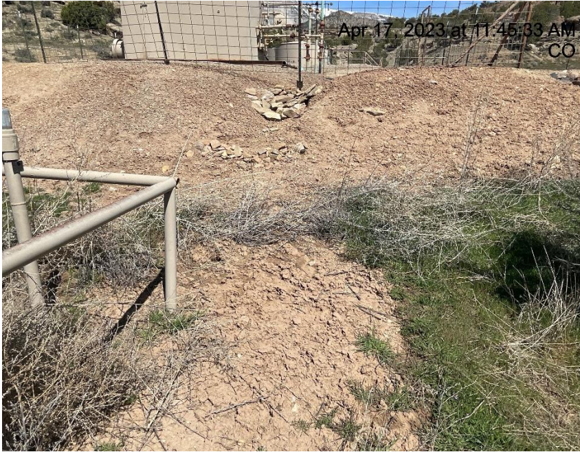
Photo # 5482 Erosion & transport of sediment off location/insufficient BMP's
