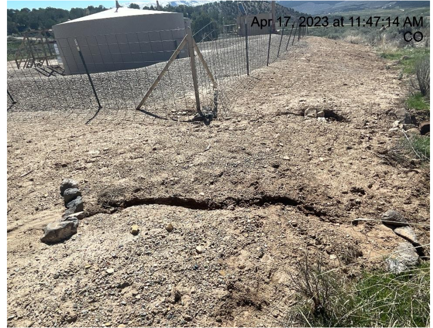
Photo # 5484 Check dams need maintenance
