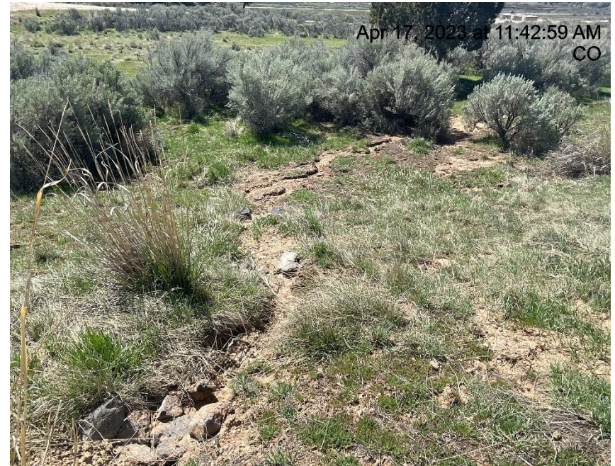
Photo # 5474 Transport of sediment off location/choking off vegetation/insufficient BMP's (SE area of location, near entrance to location)
