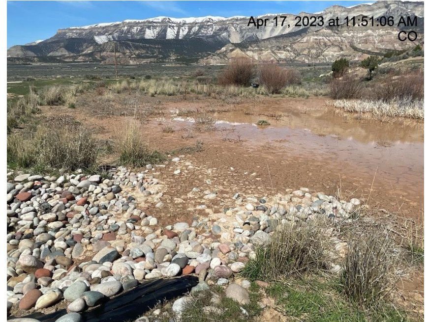
Photo # 5493 Retention Pond/BMP's need maintenance (on north side of lease road approximately 1/10 th of a mile from location)
