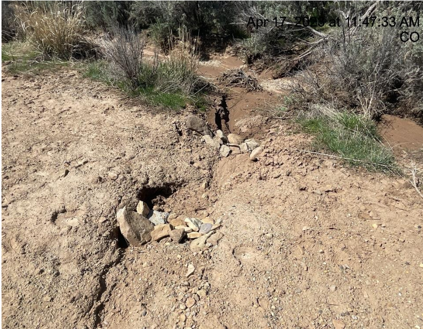
Photo # 5486 Check dams need maintenance
