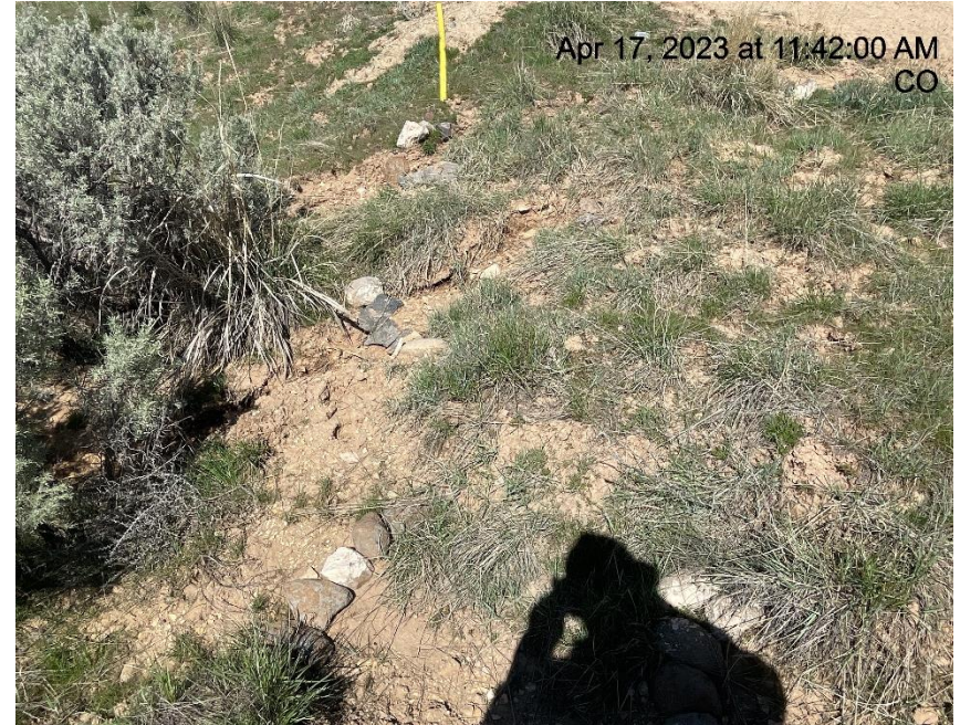
Photo # 5469 Erosion & transport of sediment off location/insufficient BMP's (SE area of location, near entrance to location)
