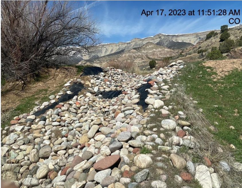
Photo # 5494 Rip Rap run needs maintenance (on north side of lease road approximately 1/10 th of a mile from location)
