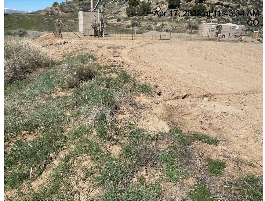
Photo # 5478 Erosion & transport of sediment off location
