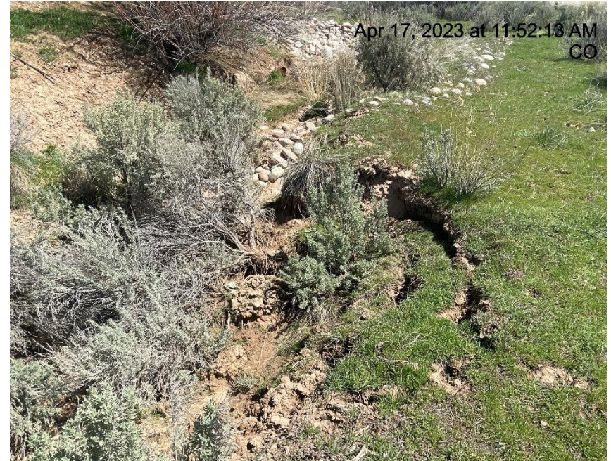
Photo # 5497 Ditch needs maintenance/insufficient BMP's/erosion of habitat (on north side of lease road approximately 1/10 th of a mile from location)
