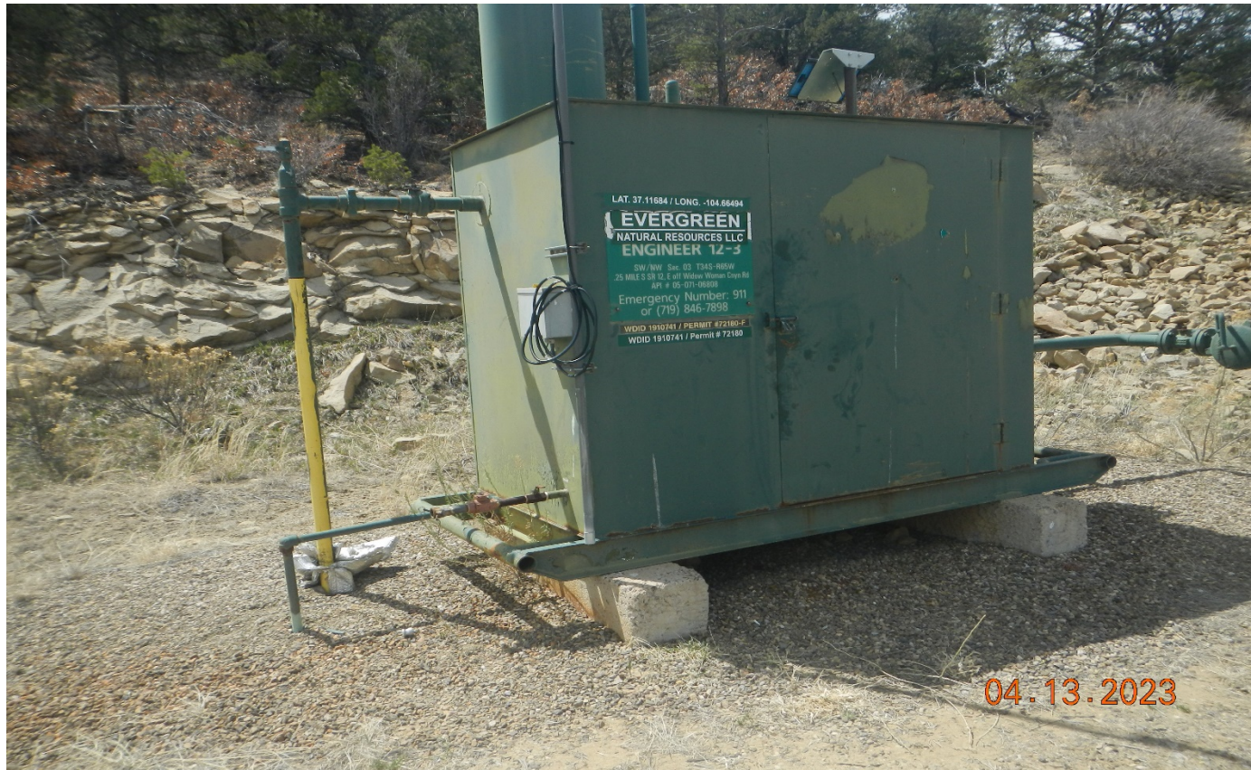
Photo 2. Well sign posted at meter shed.
