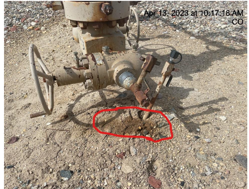
Photo # 5368 Stained soils & gravel
