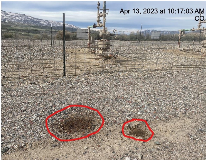
Photo # 5367 Stained soils & gravel
