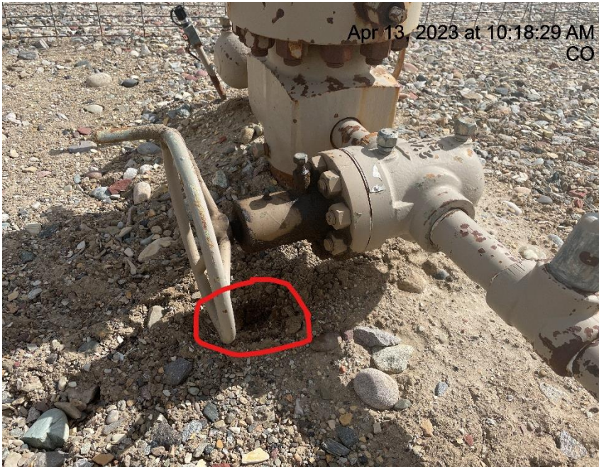
Photo # 5370 Stained soils & gravel
