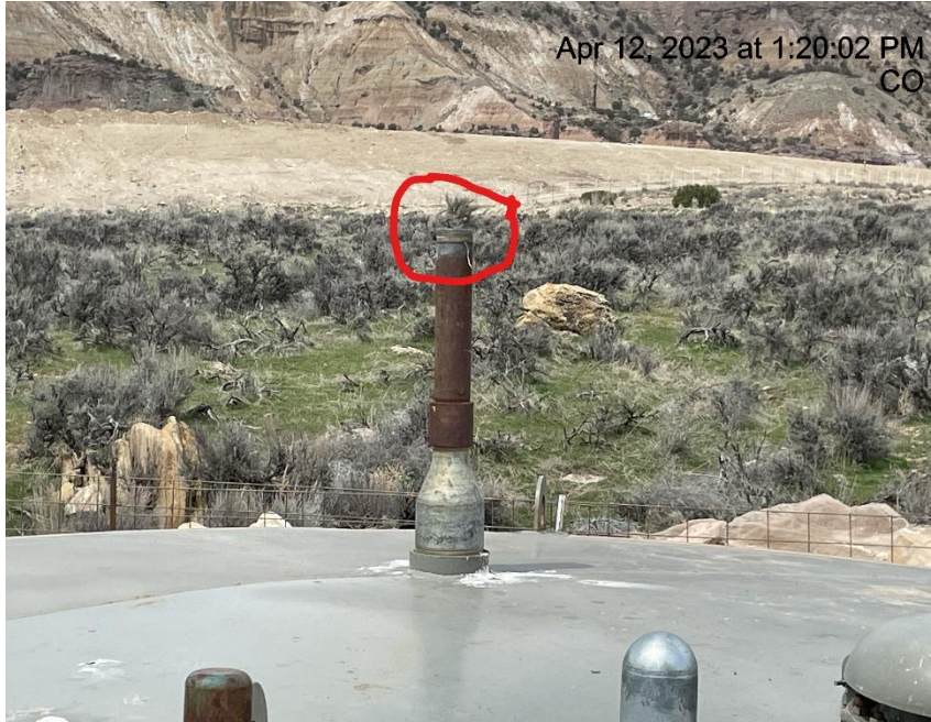
Photo # 5239 Open ended pipe on top of production tank
