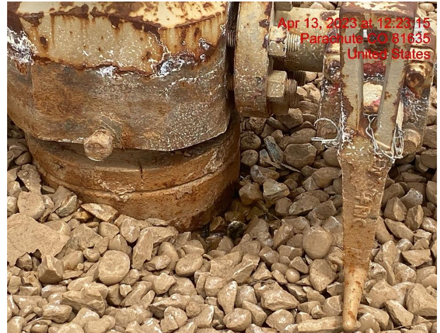
Casing Flange Leak – Photo #02157
