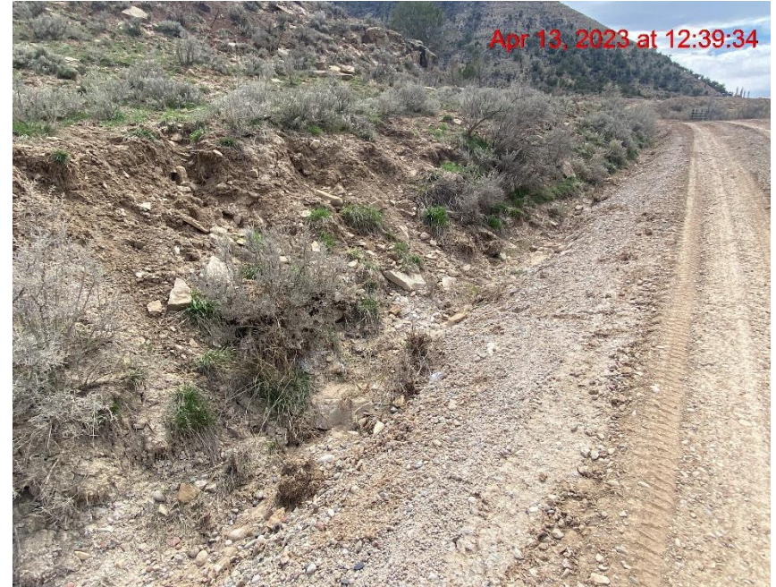
Slope Erosion into Lease Road Ditch – Photo #02178
