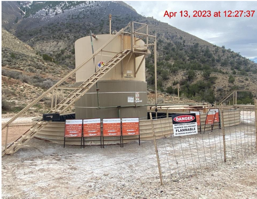
Tank Battery – Photo #02163
