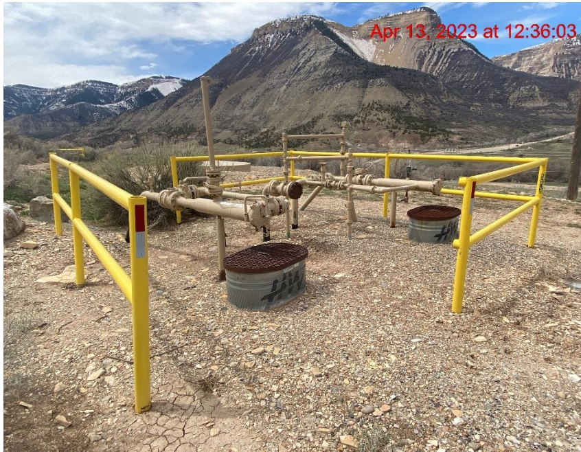
Pig Station – Photo #02172
