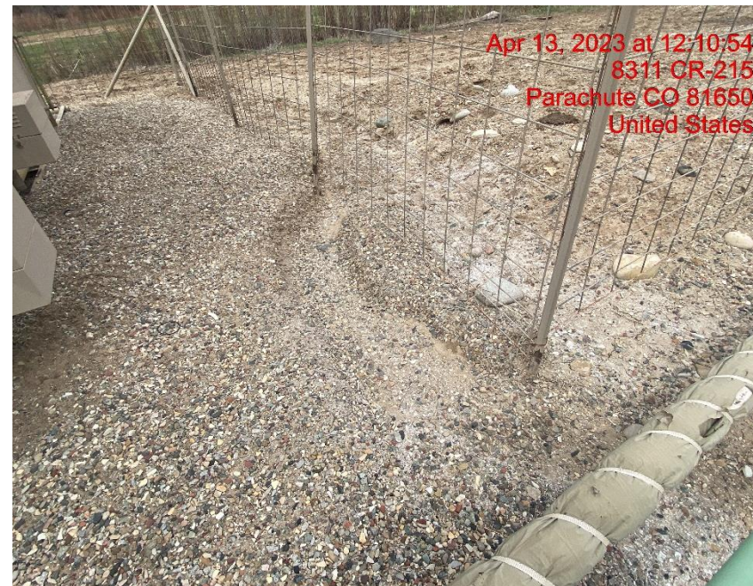
Rill Erosion – Photo #02144
