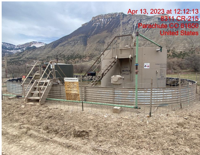
Tank Battery – Photo #02146
