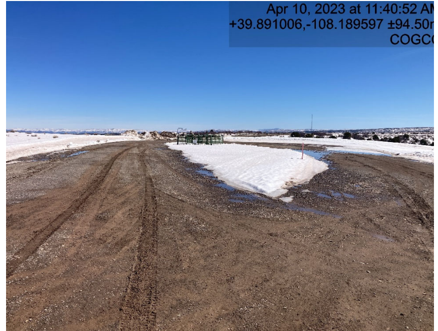
Location shows some signs of lack of stabilization
