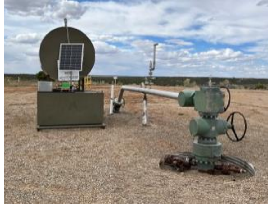
Photo #2. View of wellhead and ancillary equipment.
