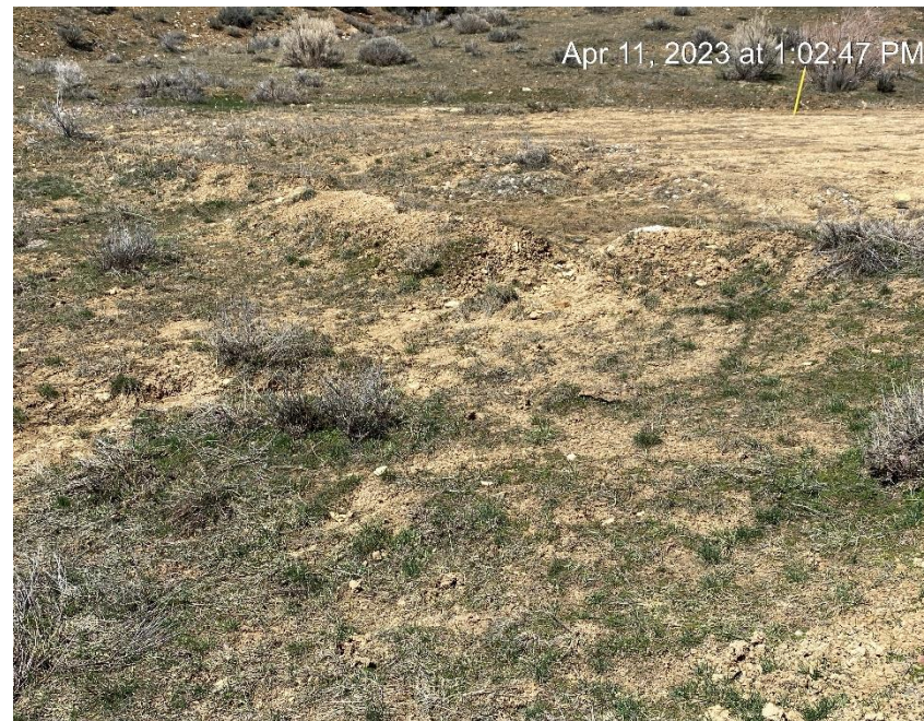
Sediment migration through berm erosion
