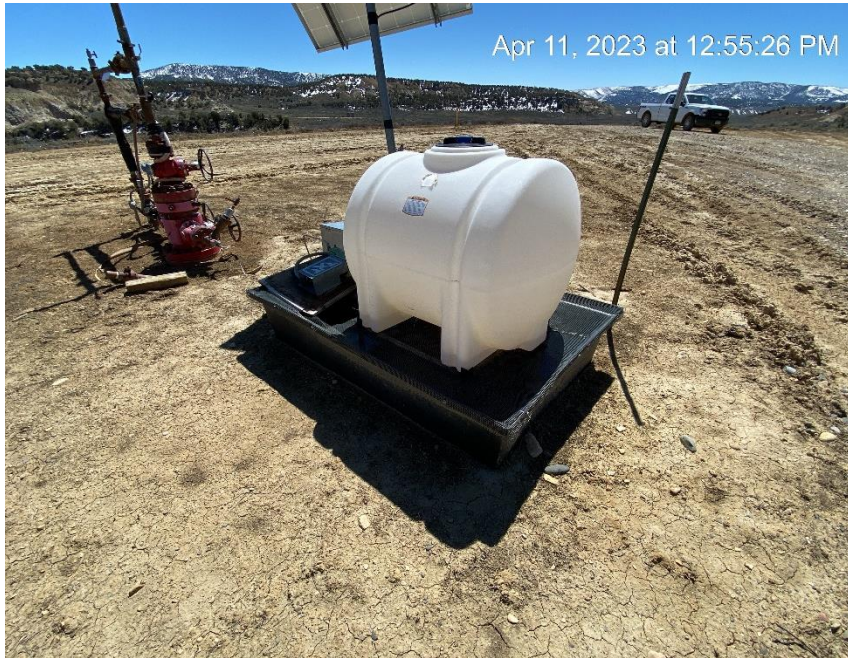
Chemical tank labels missing and/or illegible
