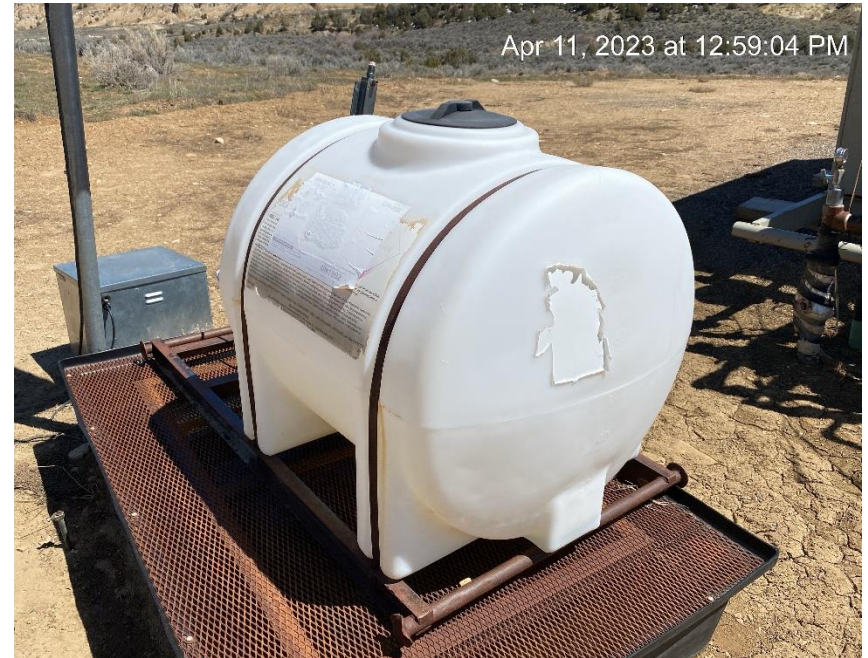
Chemical tank labels missing and/or illegible
