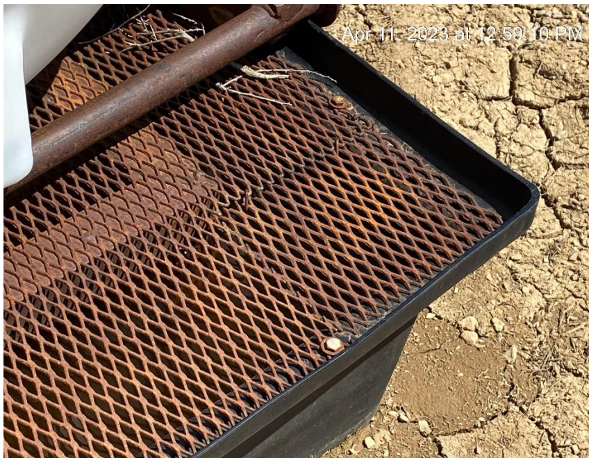
Containment full of liquid waste
