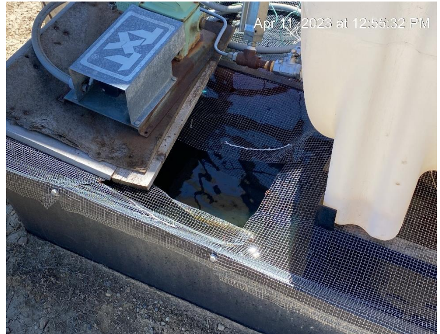
Containment full of liquid waste
