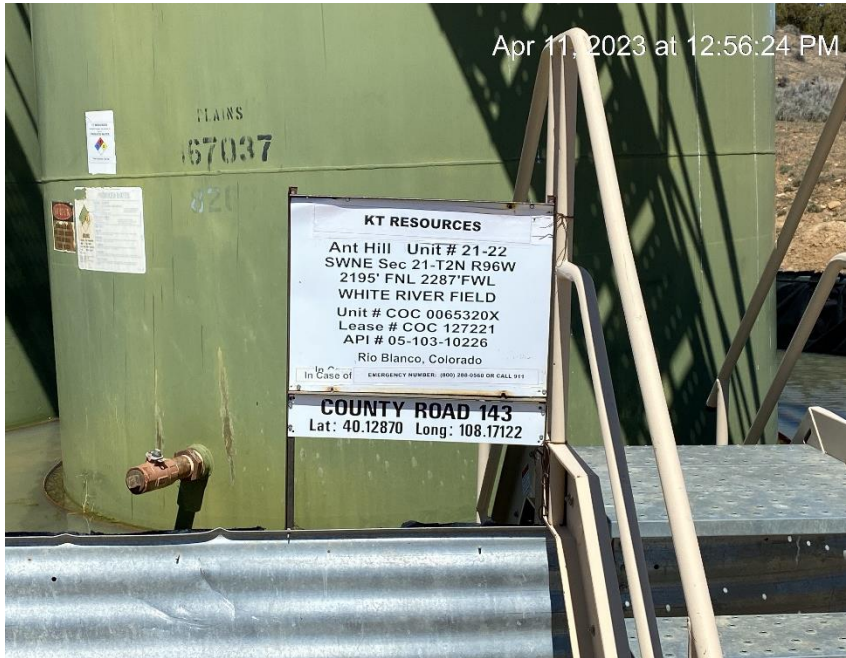
Sign at tank battery
