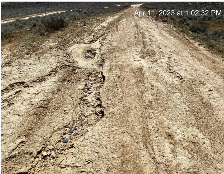
Sediment migration down lease road
