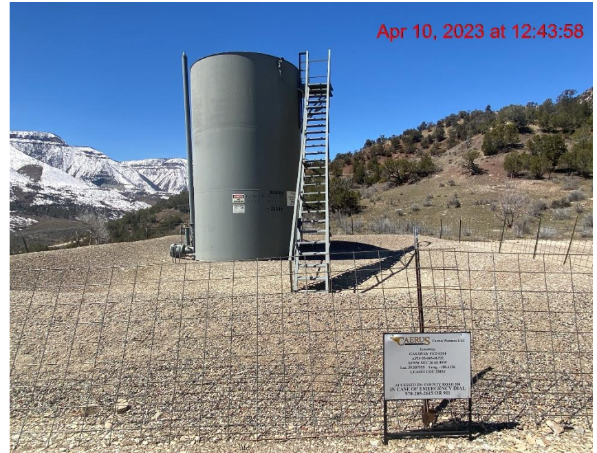
Tank Battery – Photo #02033
