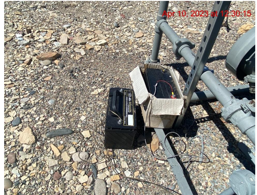
Lack of Secondary Containment – Photo #02014
