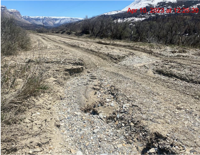
Lease Road Erosion – Photo #02005
