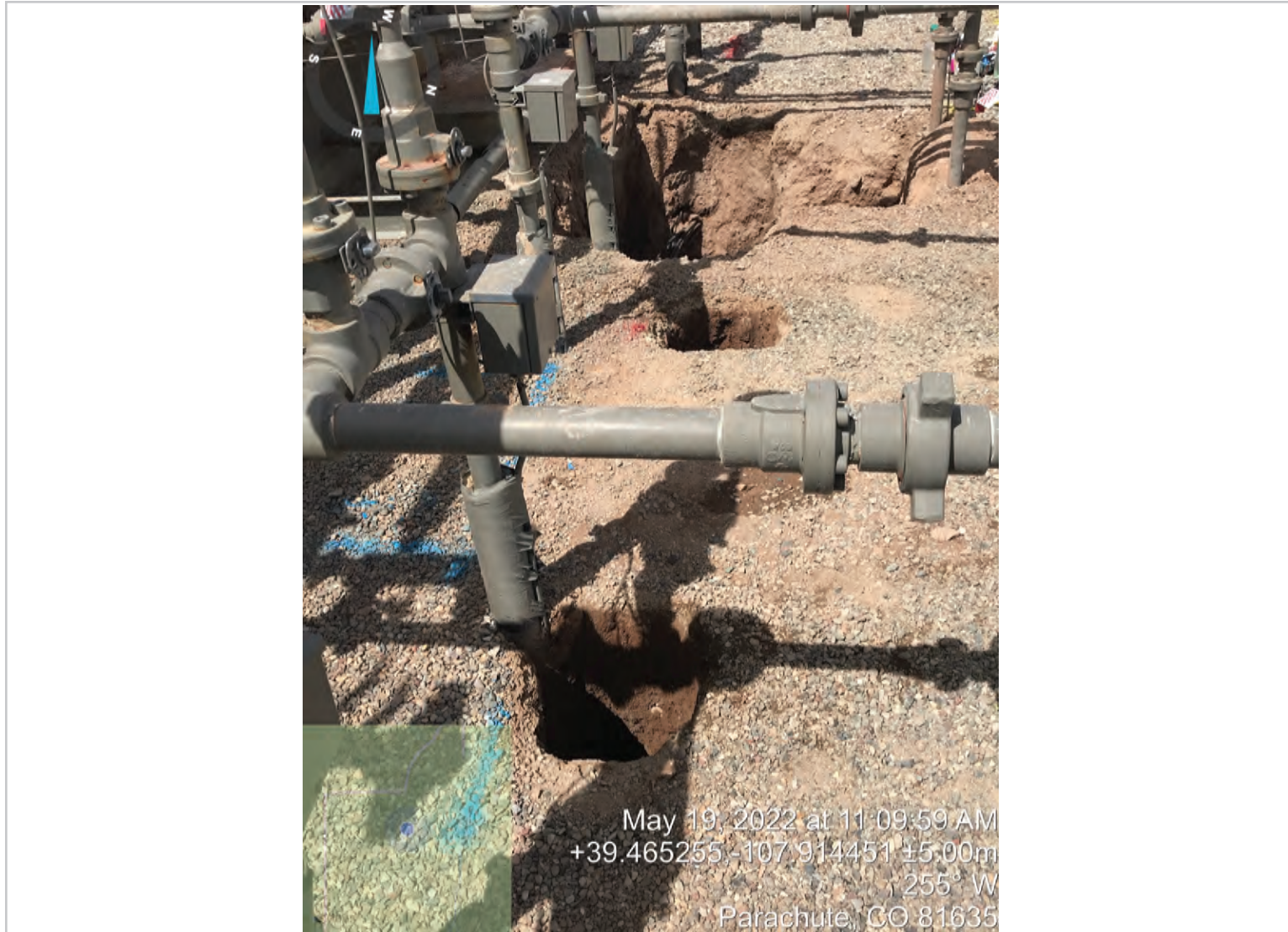
Site Delineation Potholes: View West
