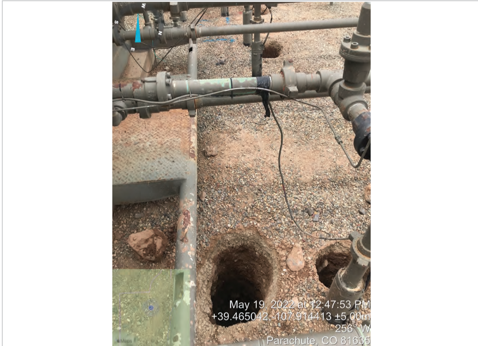
Site Delineation Potholes: View West
