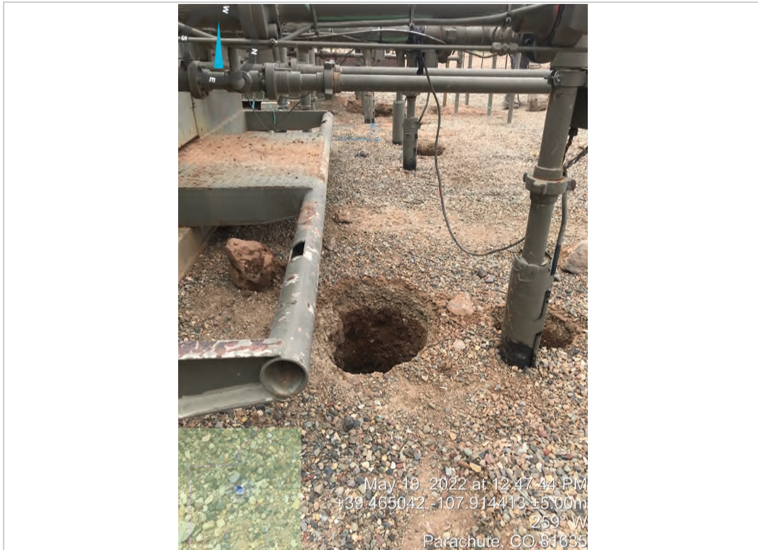
Site Delineation Potholes: View West
