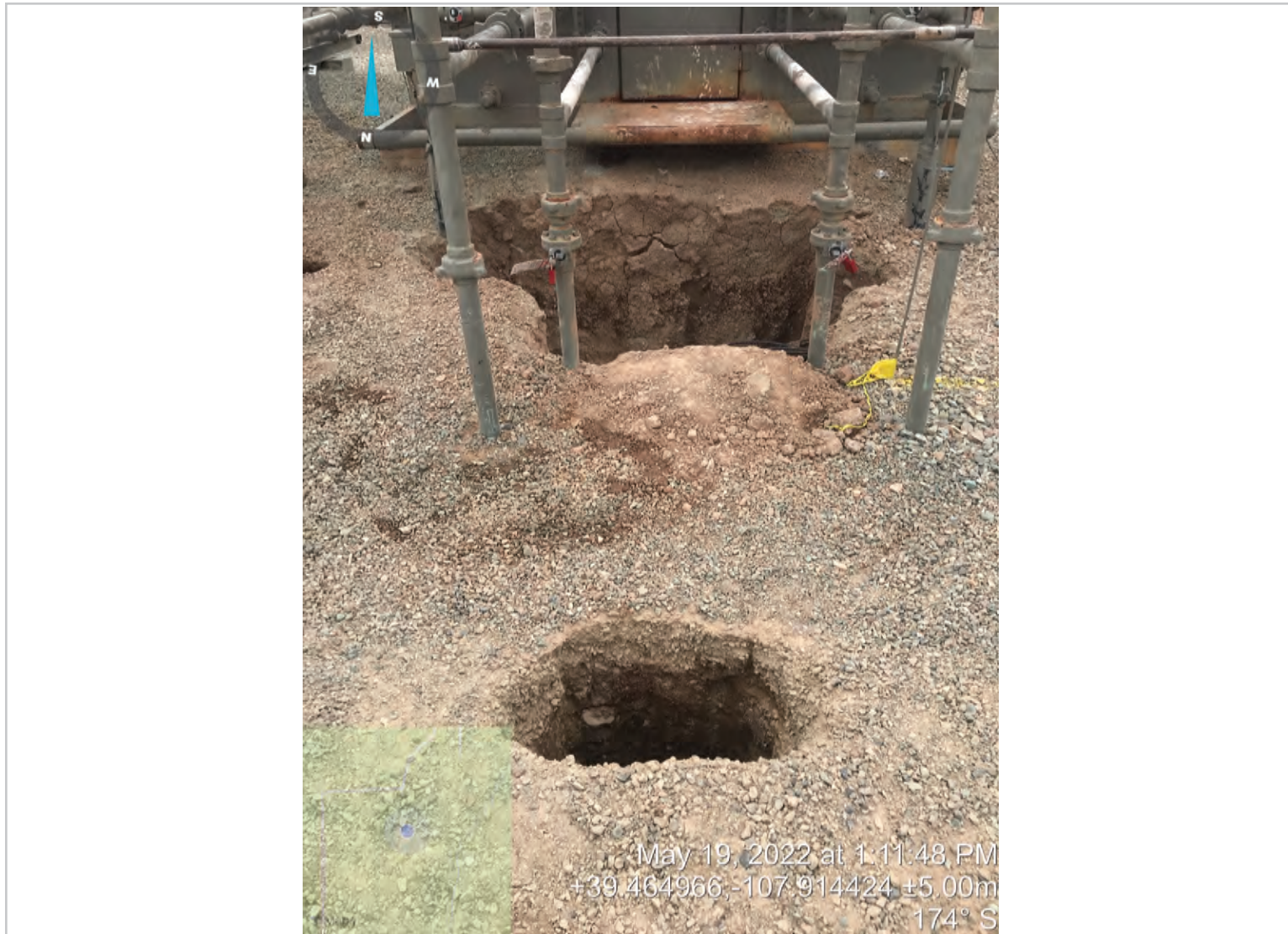
Site Delineation Potholes: View South
