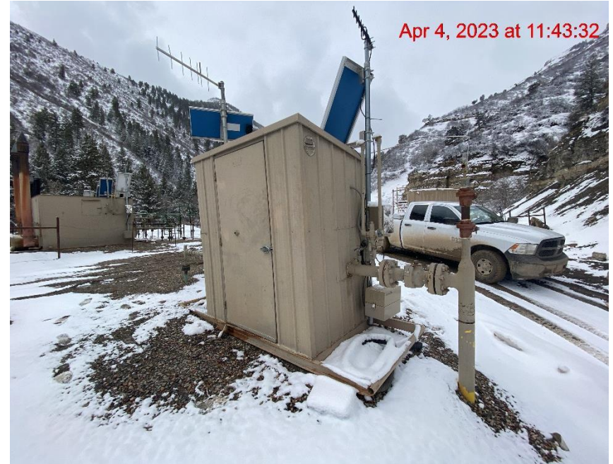
Gas Meter – Photo #01880
