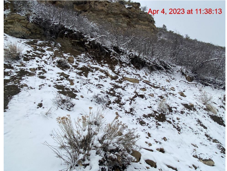
Cut Slope Erosion/Run-On – Photo #01878
