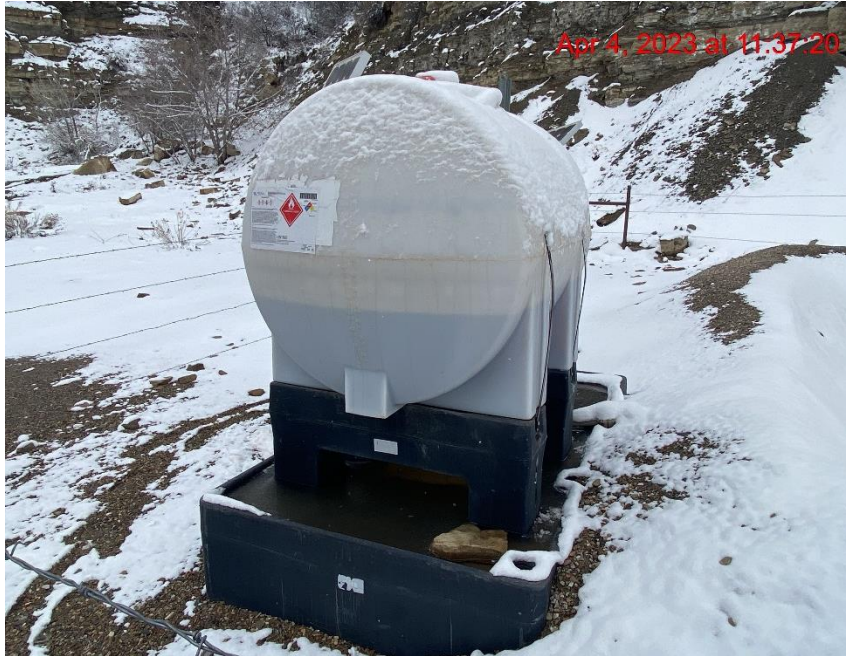
Chemical Tank – Photo #01876
