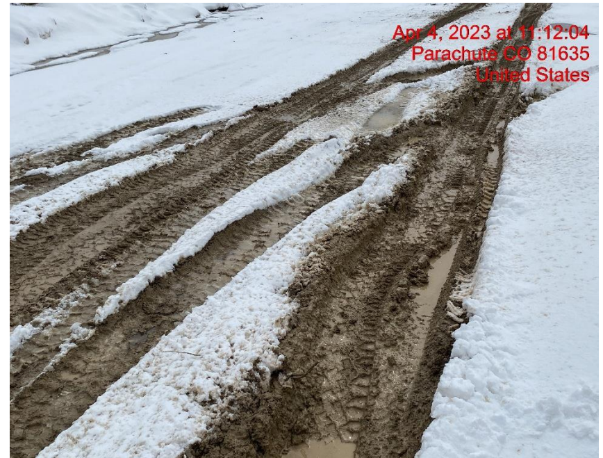
Lack of Stabilization/Inadequate Tracking BMP – Photo #01866
