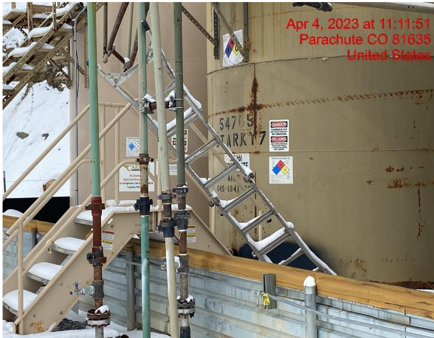
Unused Equipment (Ladder) – Photo #01865
