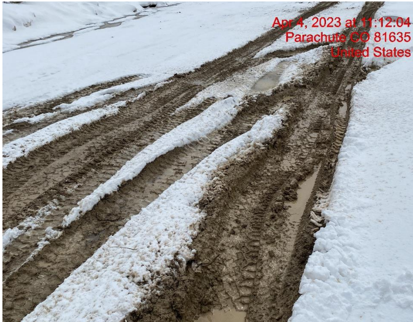
Lack of Stabilization/Inadequate Tracking BMP – Photo #01866
