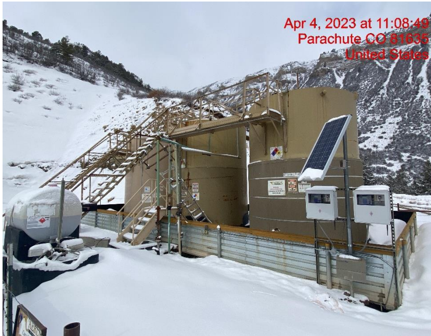
Tank Battery – Photo #01861
