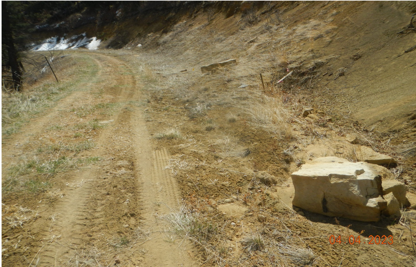
Photo 2. Facing east along the access road. There are a few culverts that are filled in with sediment and stormwater is not properly diverted that need maintenance.
