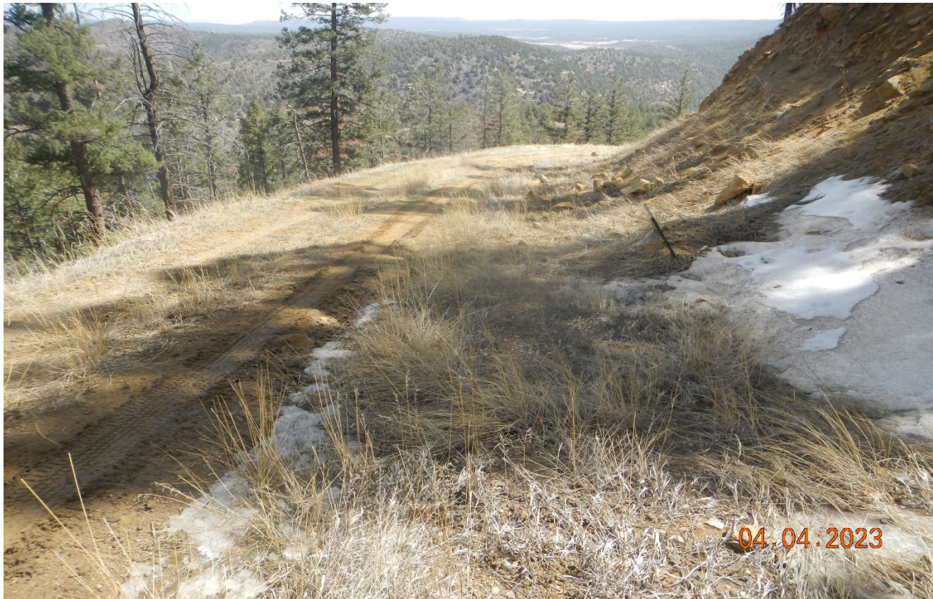
Photo 1. Facing east along the access road. There are a few culverts that are filled in with sediment and stormwater is not properly diverted that need maintenance.
