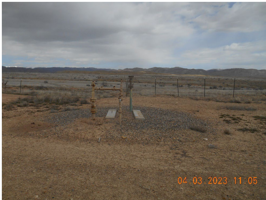
Separator risers locked out/tagged out
