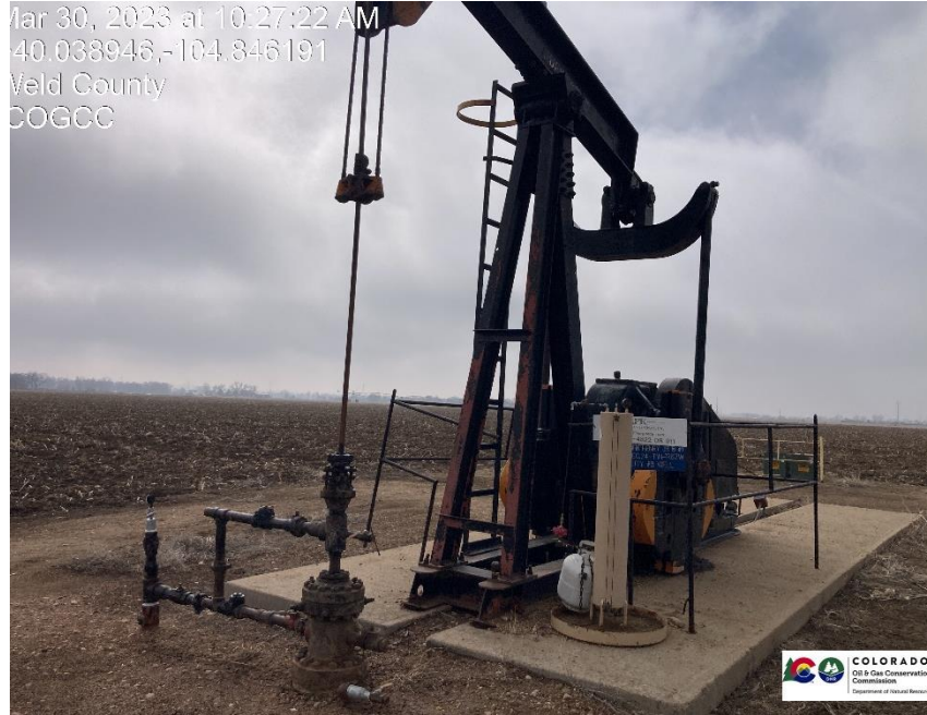
Pic 1 pump jack
