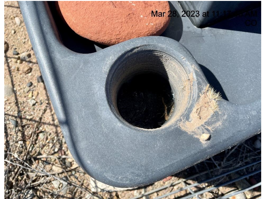
Photo # 3576 Chemical containment full/Failure to maintain chemical BMP
