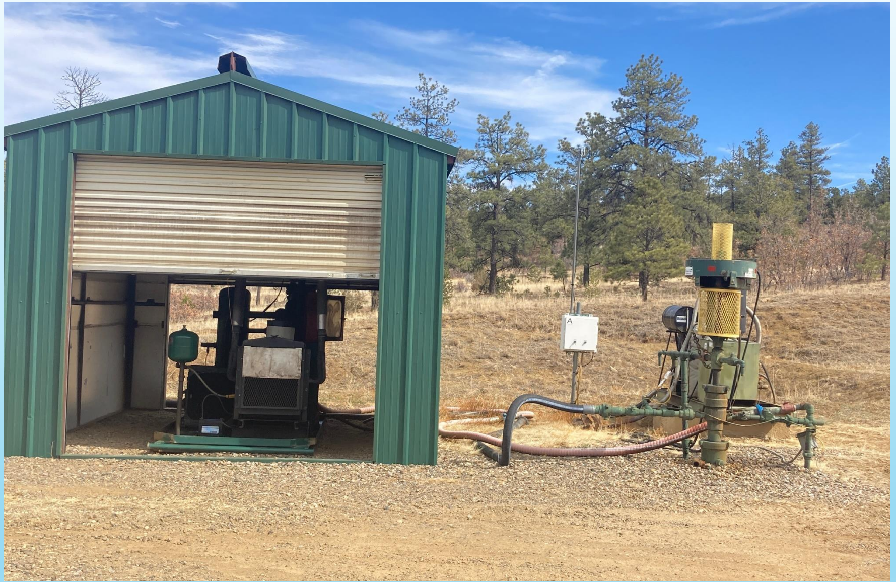
PHOTO 3: WELLHEAD AND EQUIPMENT
