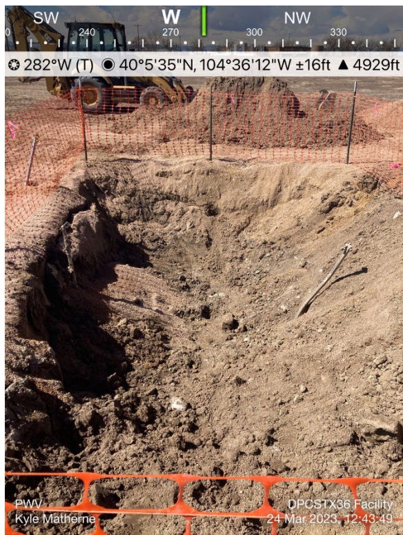
Produced Water Vessel (PWV) Footprint
