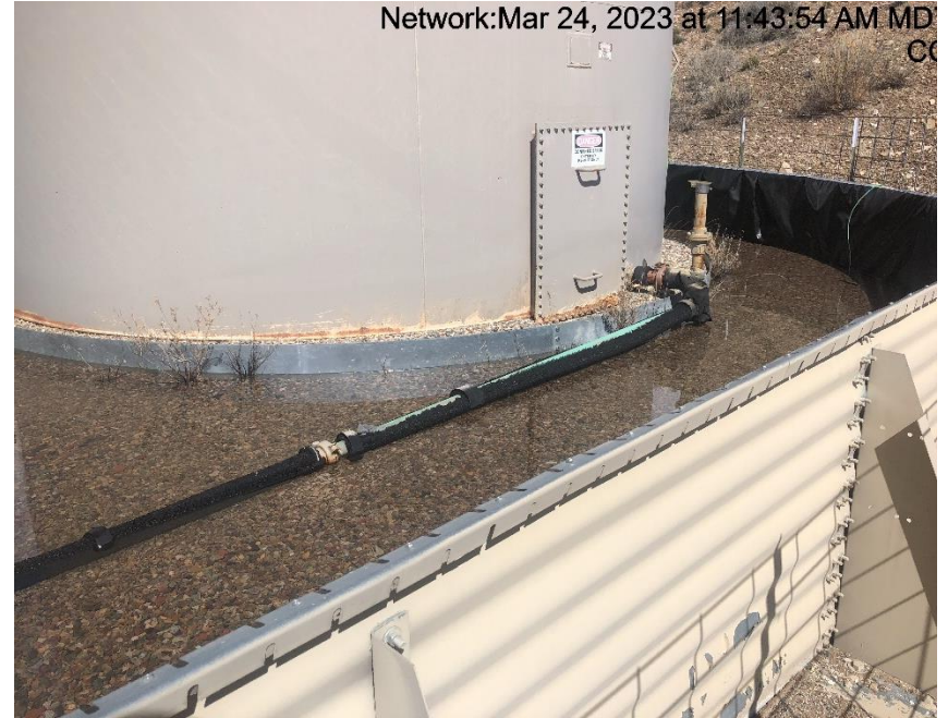
Photo #9382 Undesirable Plant Species in tank containment
