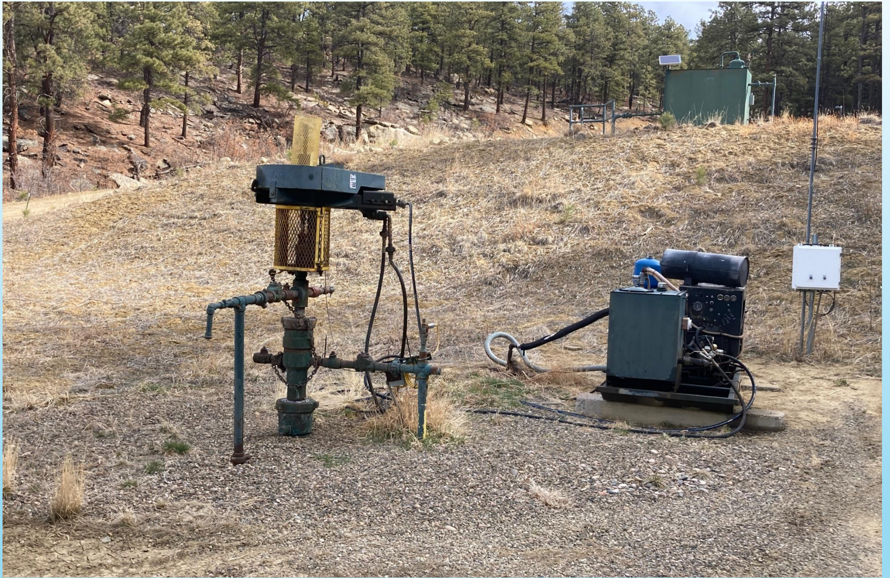
PHOTO 4: ORIGINAL WELLHEAD AND EQUIPMENT
