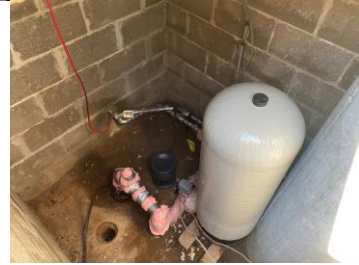
Photographs 2 & 3 35953-Gonzales Wellhead
