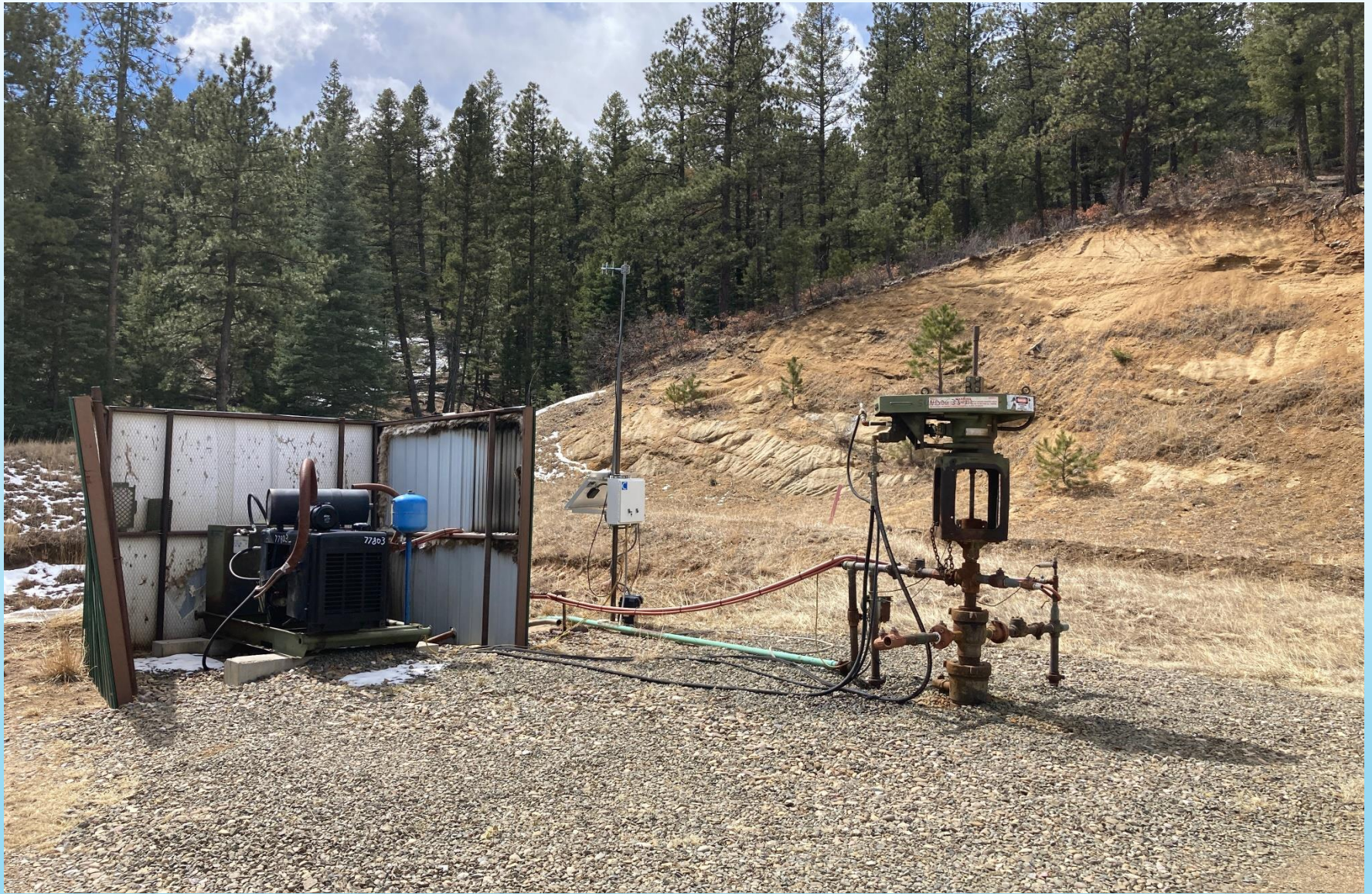
PHOTO 3: WELLHEAD AND EQUIPMENT
