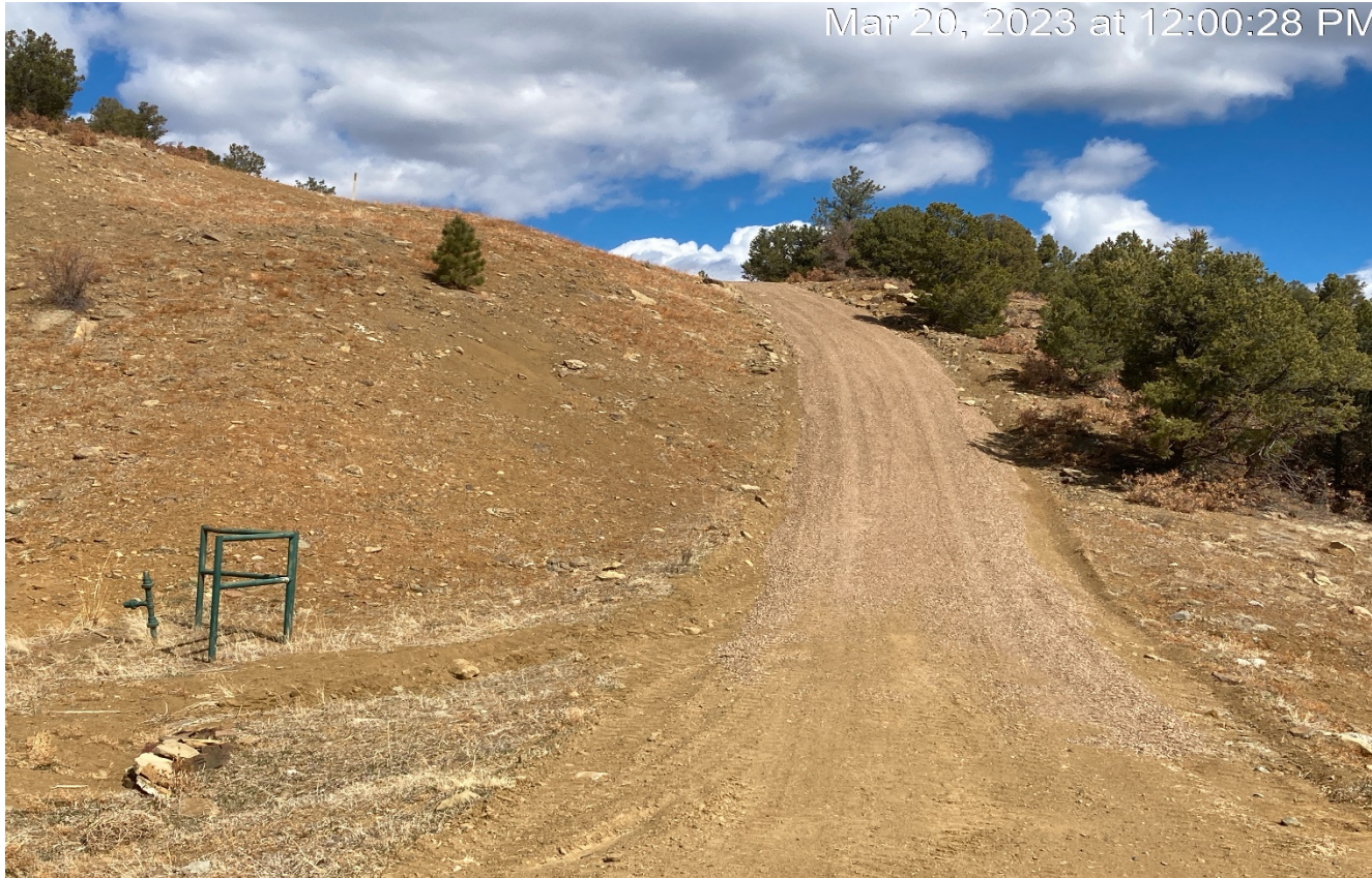
Photo 3. There has been additional gravel applied to this steep area of the road.
