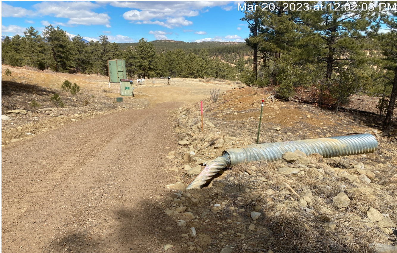
Photo 4. This damaged culvert still needs to be fixed.
