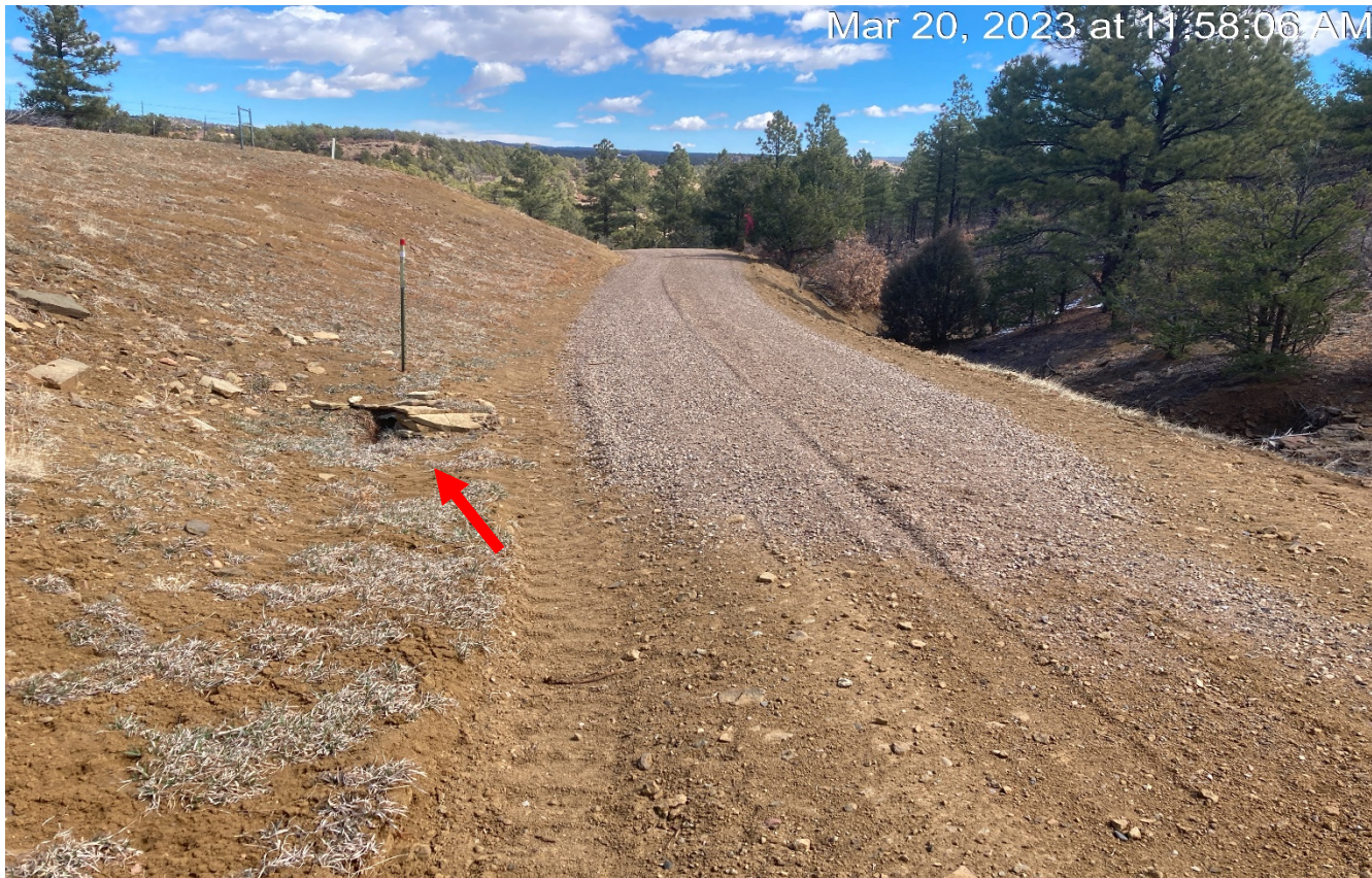
Photo 2. There has been additional gravel applied to areas of the road. Drainage to this culvert needs to be dug out better to allow proper flow to the culvert.
