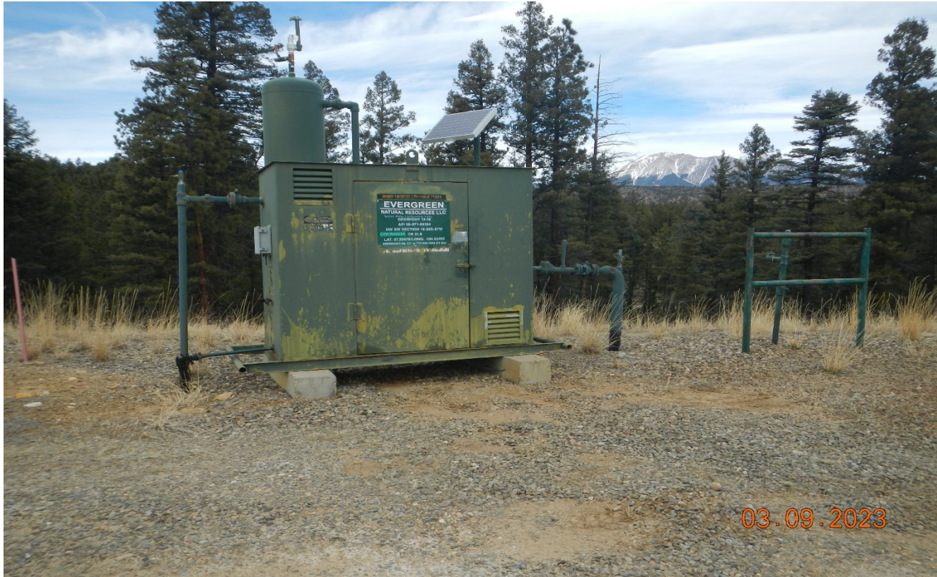
Photo 3. Sign is posted at meter shed.
