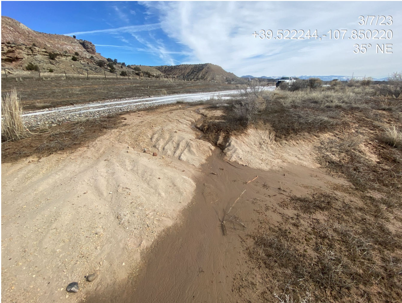
Photo 4. Photos show rill and gully erosion occurring adjacent to the access road.
