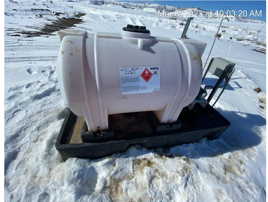
Chemical tank, containment empty
