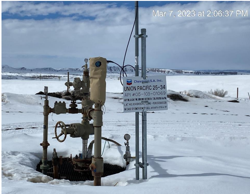
Wellhead from West side of location
