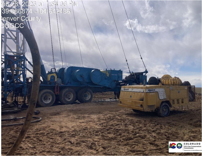
Pic 3 Rig, heater
